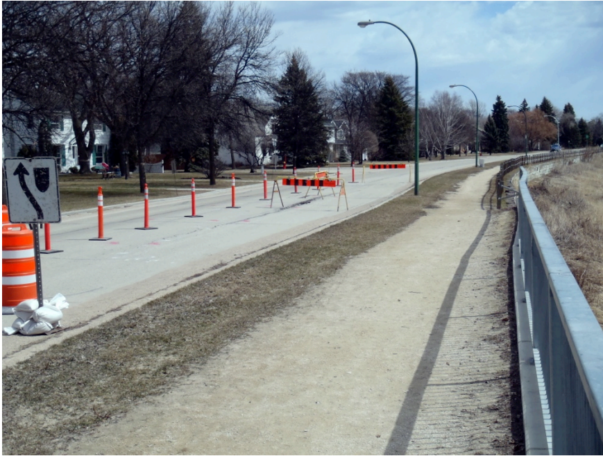
Lyndale Drive – Road failures
