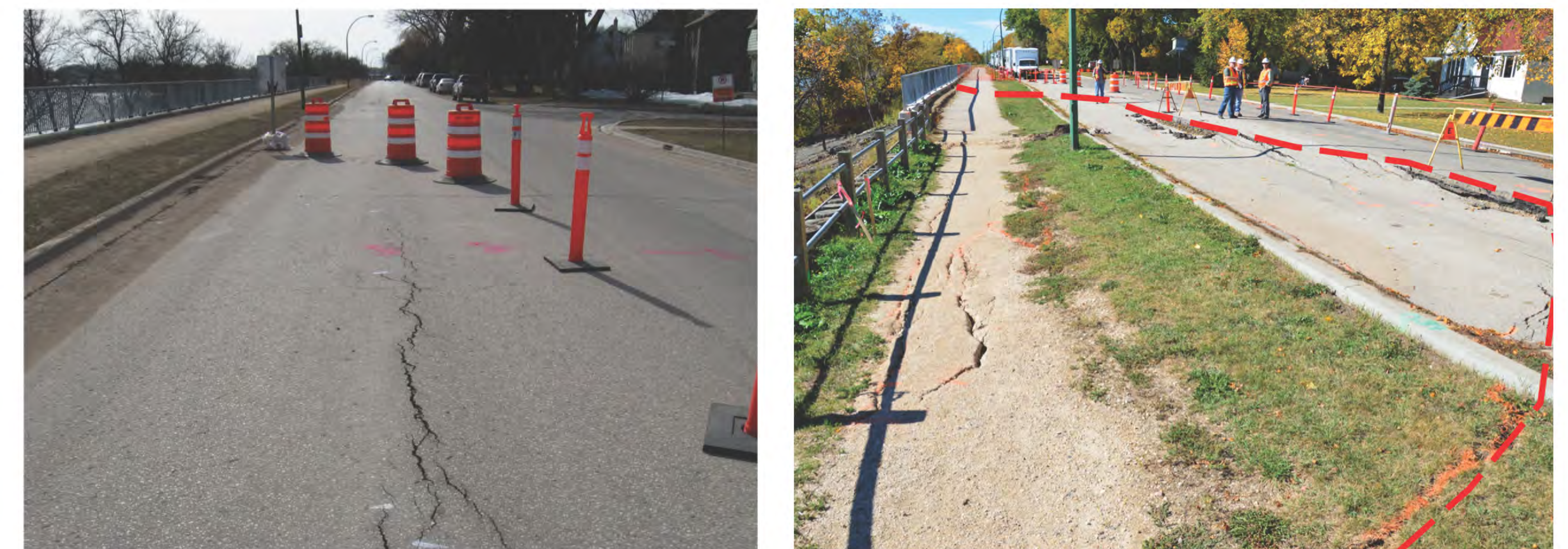
RIVERBANK INSTABILITY - MONCK TO TACHE
