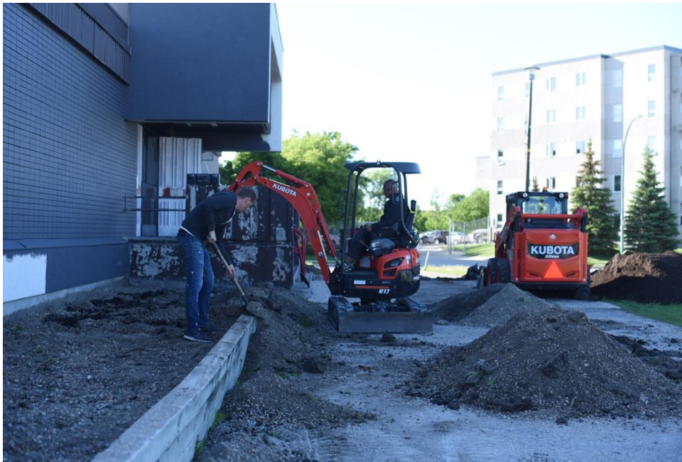
Tracy Jensen with Lawson Sales along with a volunteer remove gravel from the raised beds at the arena in preparation for installing garden soil.
