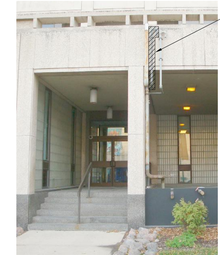
NOTE: PHOTO TAKEN OUTDOORS AT STREET LEVEL. PHOTO SCALE: NTS EXTERIOR RELIEF VENT
