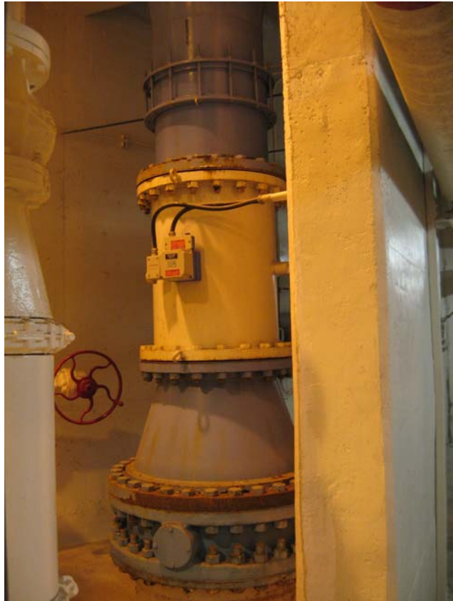
Figures 10.2: Secondary Clarifier Influent Pipeline and Flow Meter
