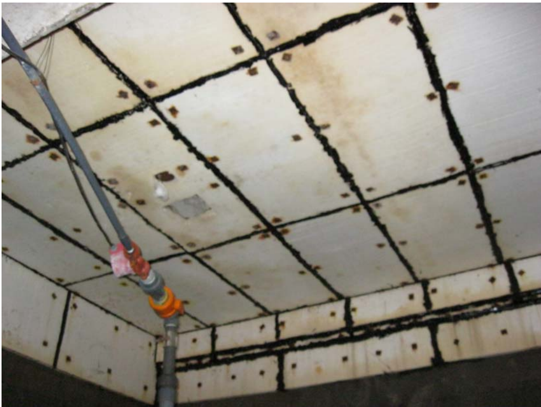
Wilkes Reservoir Valve Pit B – Ceiling above 1200 millimetre Gate Valve
