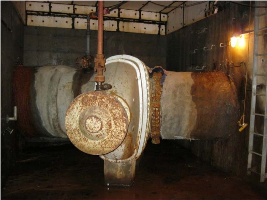
Wilkes Reservoir Valve Pit B – 1200 millimetre Gate Valve to be removed.
