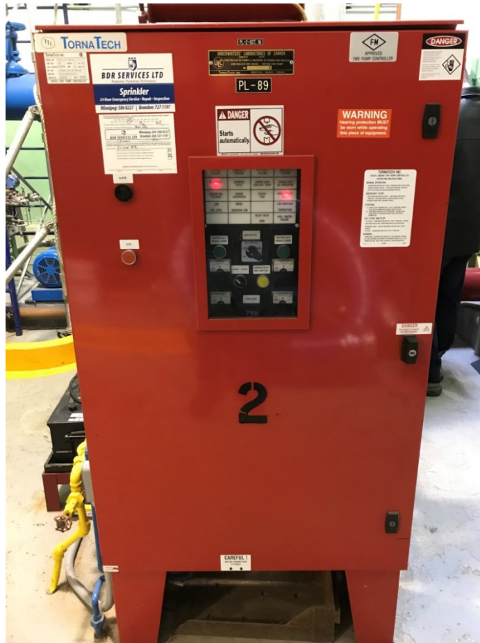
Photo 31 – Fire Pump 2 Control Panel
