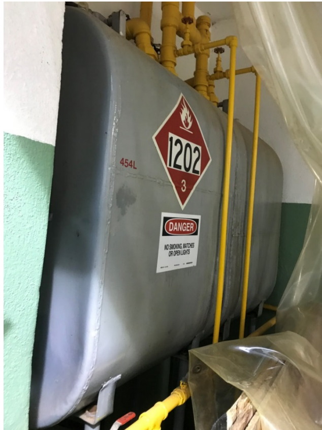
Photo 14 – Diesel Fuel Tanks
