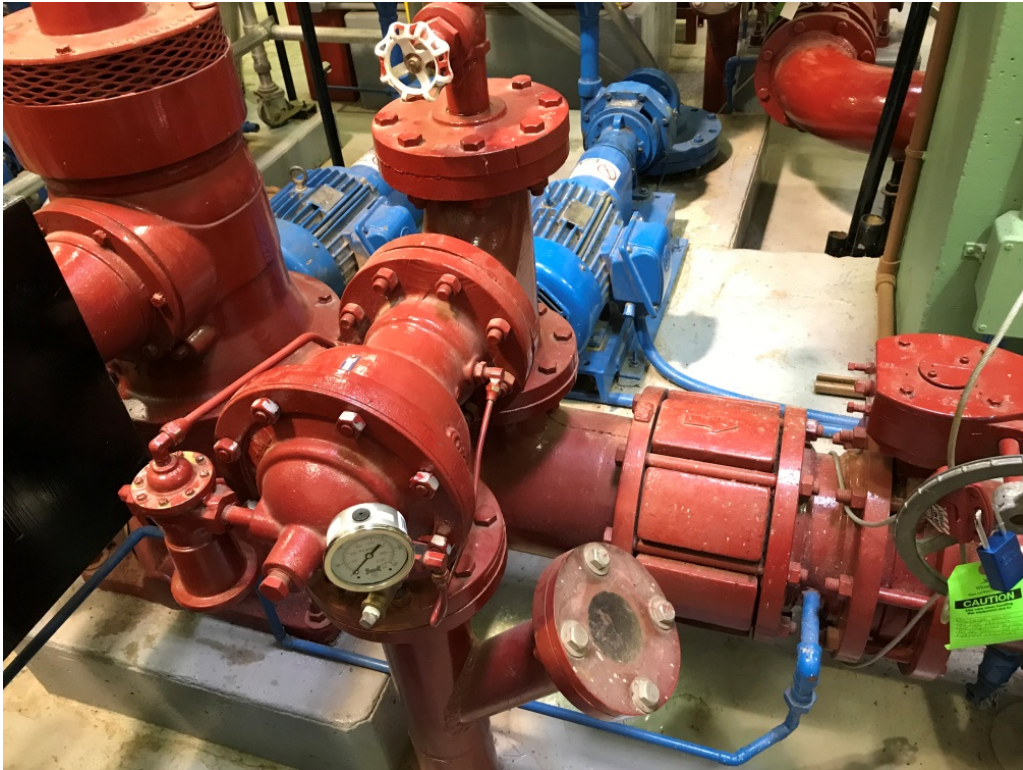
Photo 25 – Fire Pump 2 Discharge Piping
