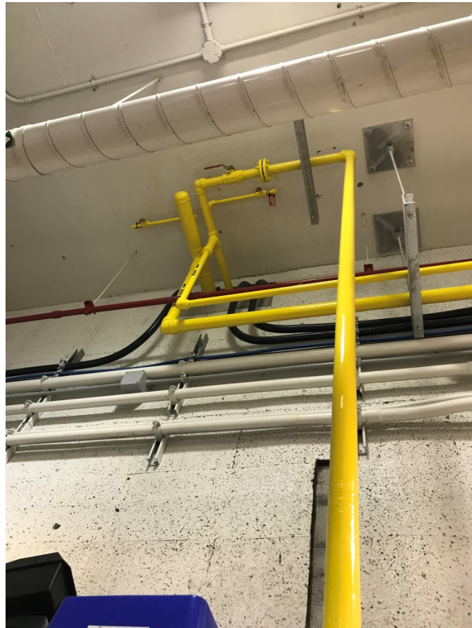
Photo 20 – Pump house Diesel Fuel Line
