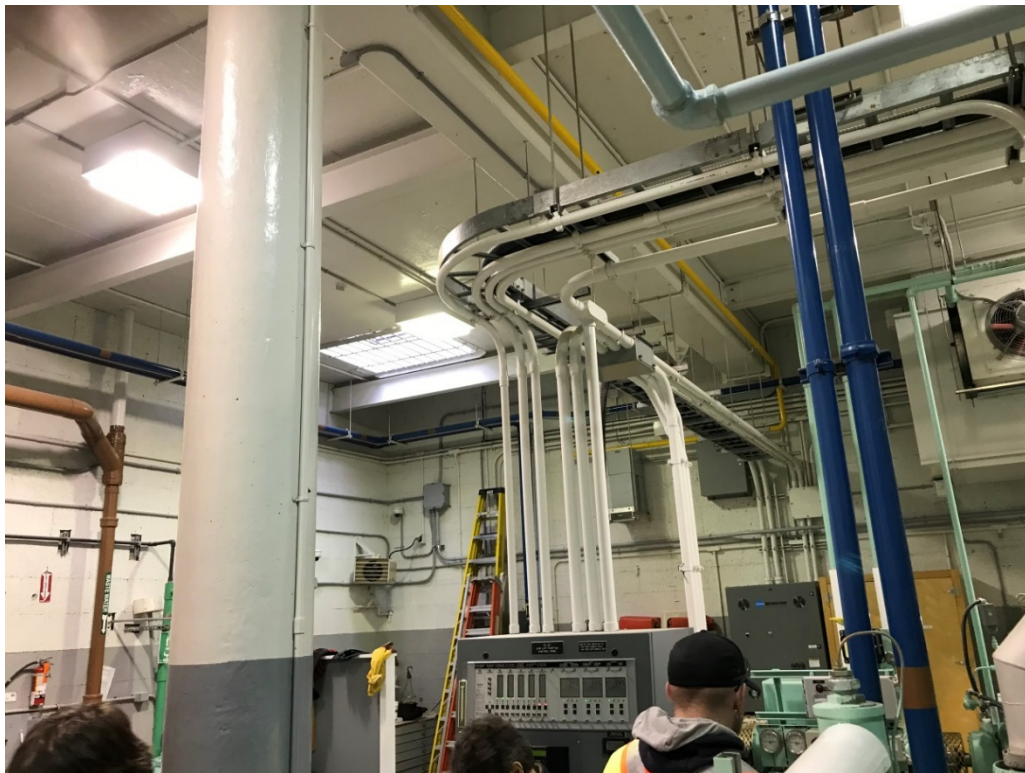
Photo 18 – Pump house Diesel Fuel Line
