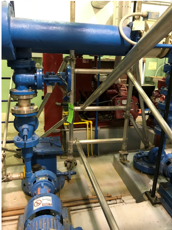
Photo 17 – Fire Pump 1 Diesel Fuel Lines
