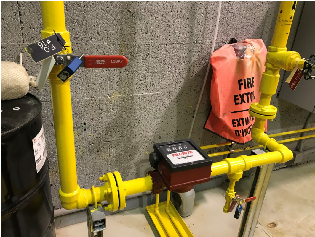
Photo 19 – Pump house Diesel Fuel Line
