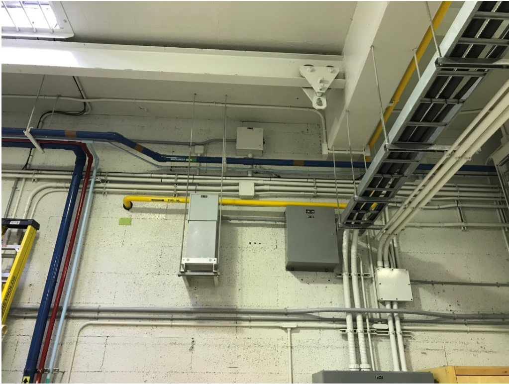
Photo 21 – Pump house Diesel Fuel Line
