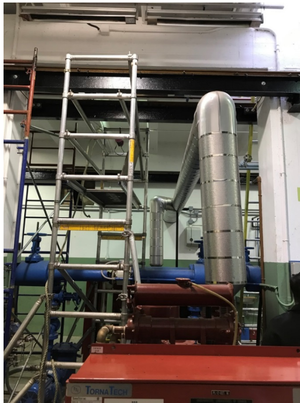
Photo 12 – Fire Pump 1 and 2 Exhausts
