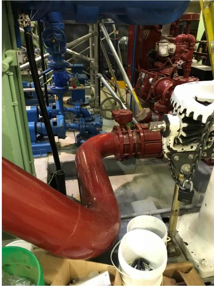
Photo 27 – Fire Pump 1 Discharge Piping
