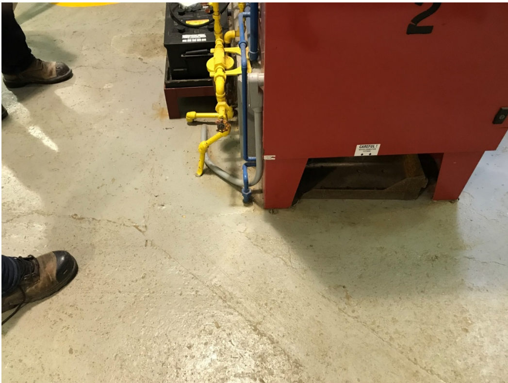
Photo 16 – Fire Pump 2 Diesel Fuel Lines
