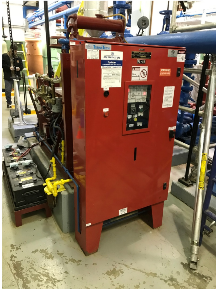
Photo 29 – Fire Pump 1 Control Panel
