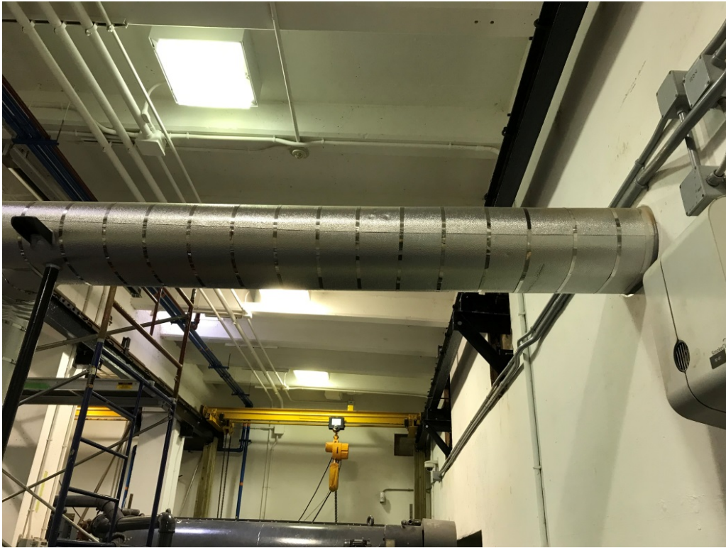
Photo 13 – Fire Pump 1 and 2 Exhausts
