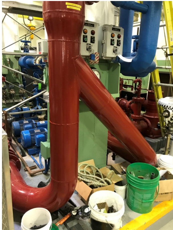
Photo 24 – Common Discharge Piping
