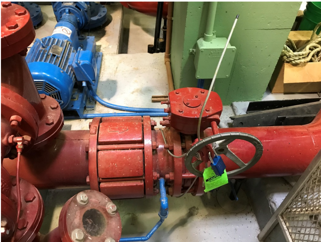
Photo 26 – Fire Pump 2 Discharge Piping
