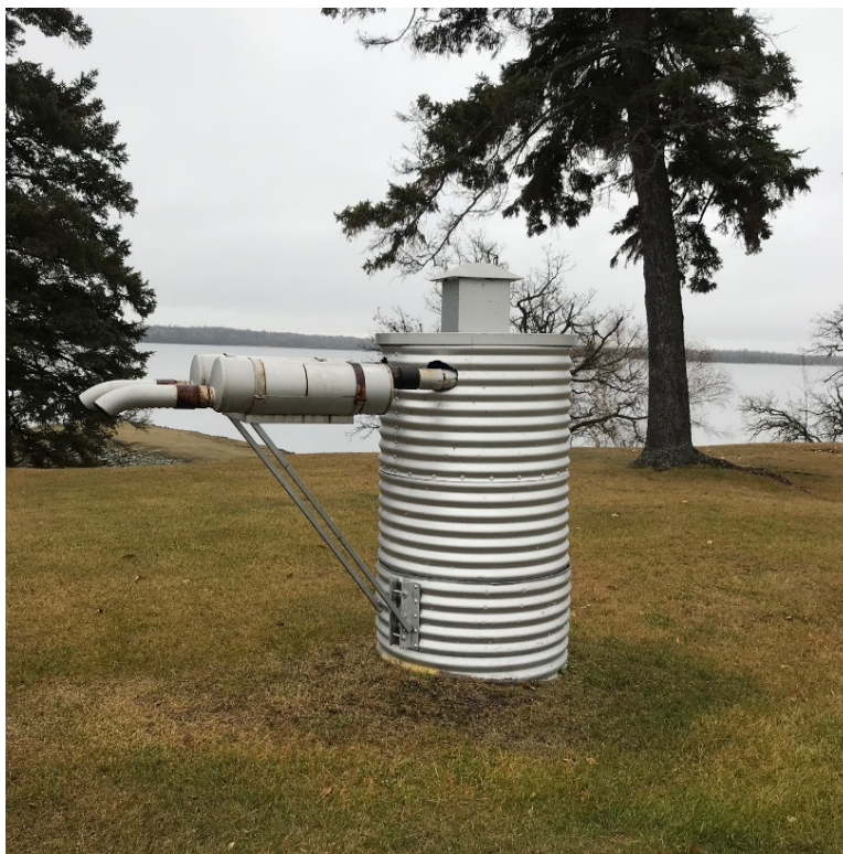
Photo 32 – Fire Pump Engine Silencers to be removed.
