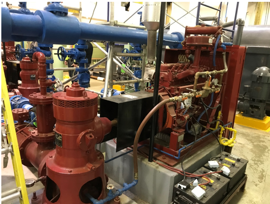
Photo 28 – Fire Pump Discharge Piping
