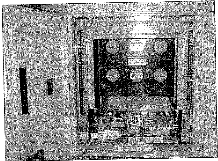
Figure 37. Ring Type CTs with Shutters Closed and CT Barrier in Place.
