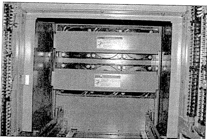
Figure 39. Primary Disconnects Behind the Closed Shutter.
