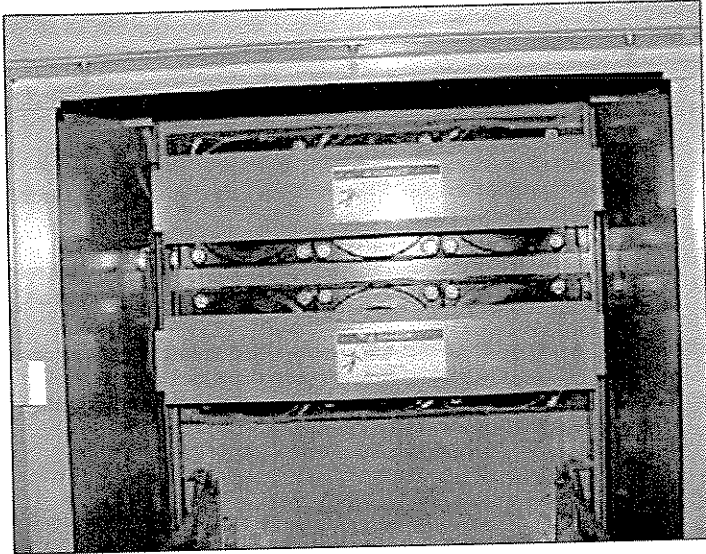
Figure 35. Automatic Shutters - Ring Type CTs with Shutters Closed and CT Barriers Removed.
