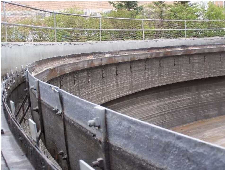
Photo 2-2 Effluent Weir & Scum Baffle
