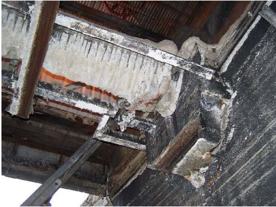
Photo 2-1 Scum Trough Discharge Box
