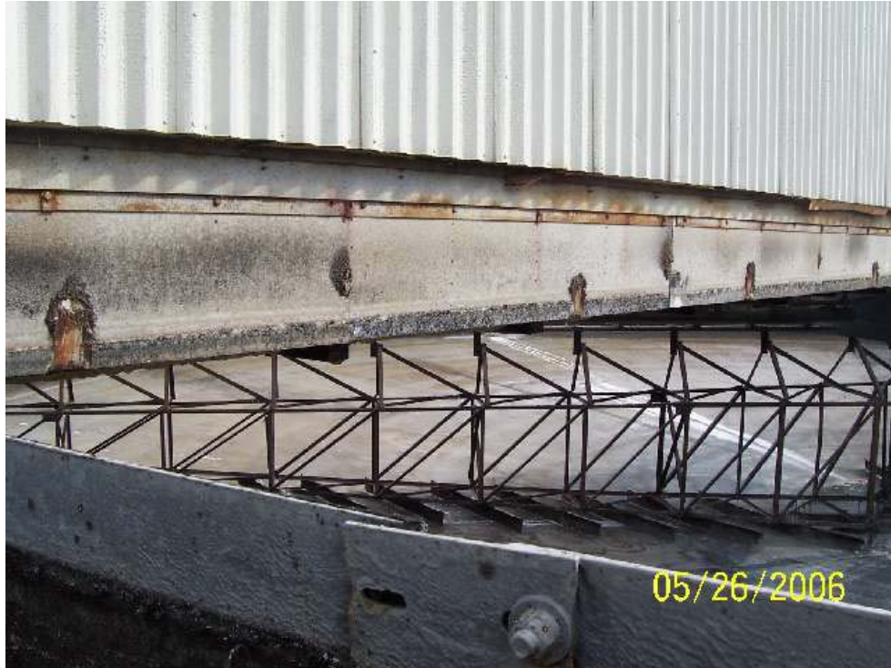
Photo 3-7 Walkway Enclosure Hinged Scum Blade Access Panels
