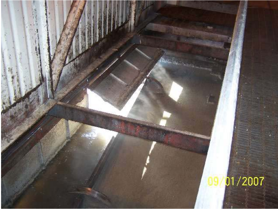
Photo 3-17 Walkway Enclosure Hinged Scum Blade Access Panels
