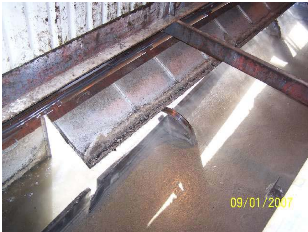
Photo 3-16 Walkway Enclosure Hinged Scum Blade Access Panels
