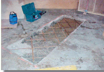
Prepare the area to be repaired in accordance with industry (ICRI) guidelines.
