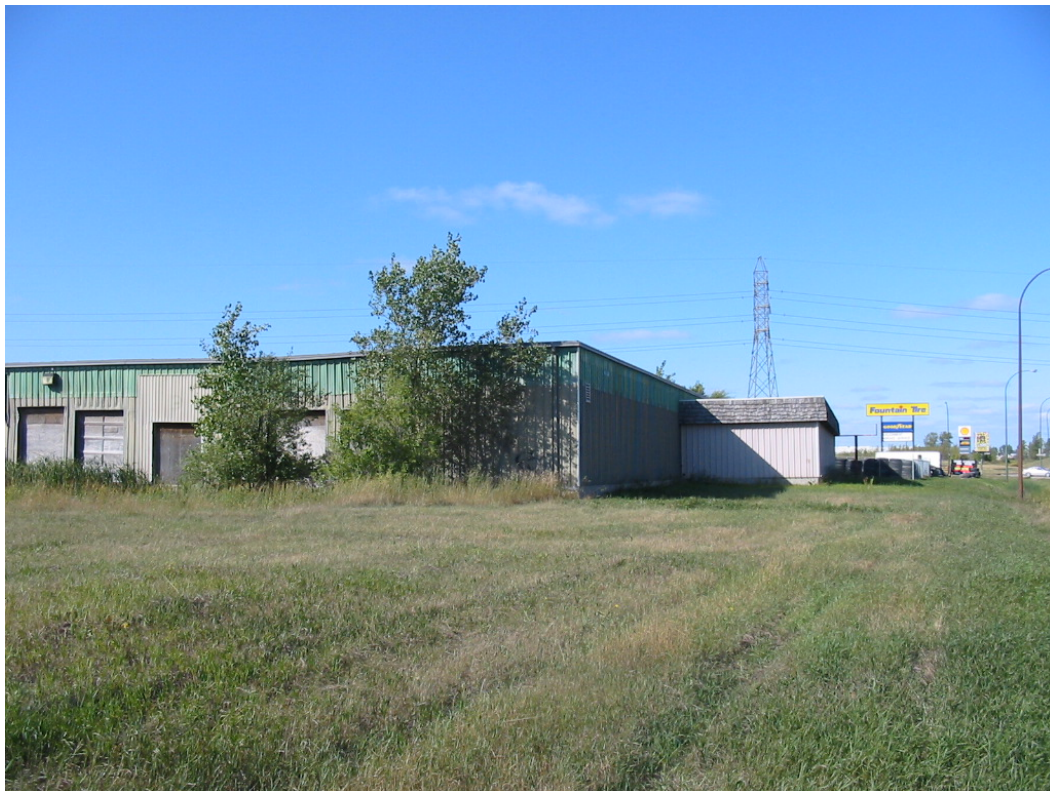
33 Fournier St – View from Lagimodiere Blvd along East Side of building (from south)
