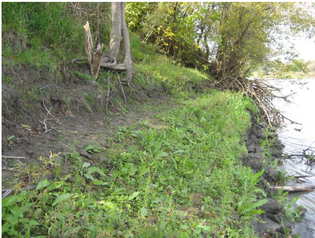
PHOTO 2 – SHORELINE EROSION ALONG ST. VITAL PARK SIDE OF RED RIVER AT THE PIPE CROSSING
