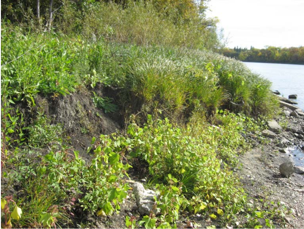
PHOTO 3 – SHORELINE EROSION ALONG SOUTH DRIVE PARK SIDE OF RED RIVER AT PIPE CROSSING
