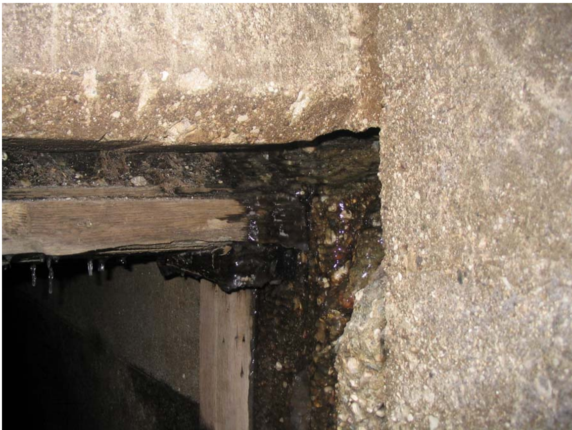
Mile 50.31 Lower Construction Joint
