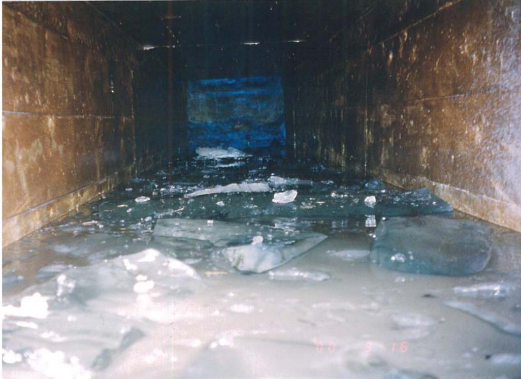
Mile 53.75 Drainage Siphon Lower Box at S. End Looking N. (Note: Good condition)
