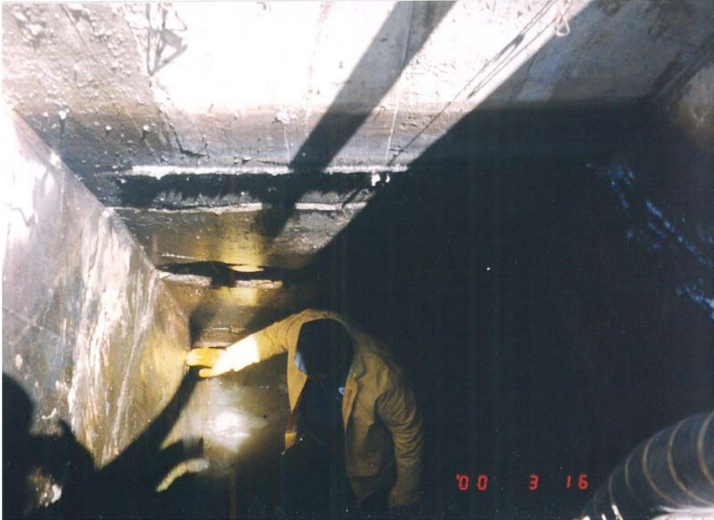
Mile 53.75 Drainage Siphon S. Side Looking Down S. Throat (Note 2 Transverse Cracks)
