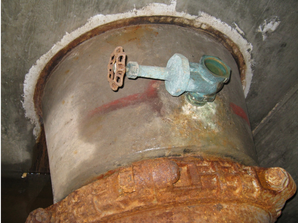
Typical Small Diameter Valve Condition
