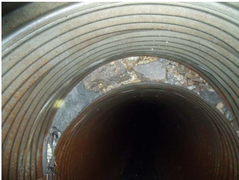
Figure 3: Large displaced joint (Probable location of sink hole) looking downstream
