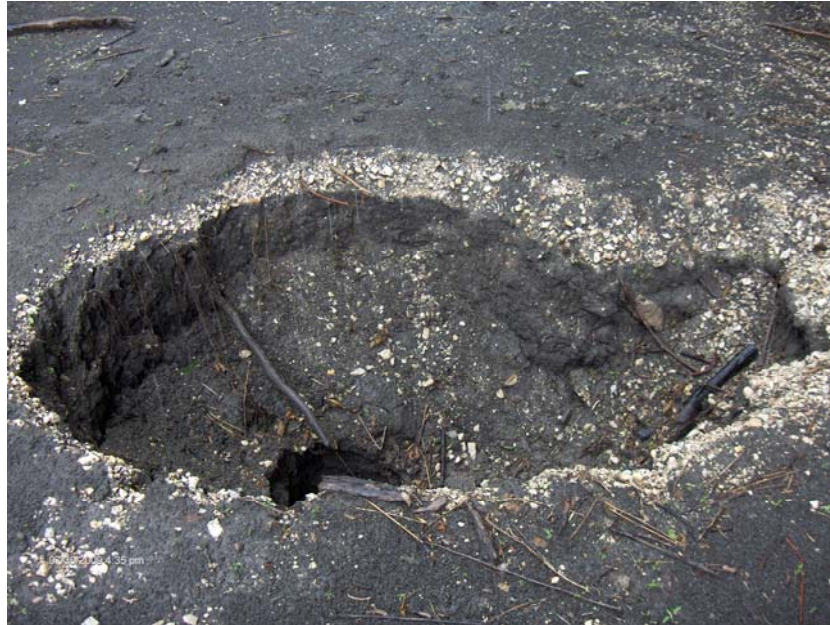
Figure 1: Sinkhole above Outfall RR-7
