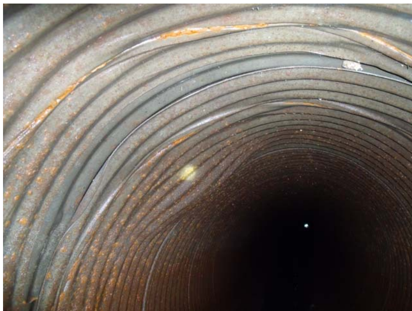
Figure 9: Deformed sewer at Joint – Looking at bulge in pipe
