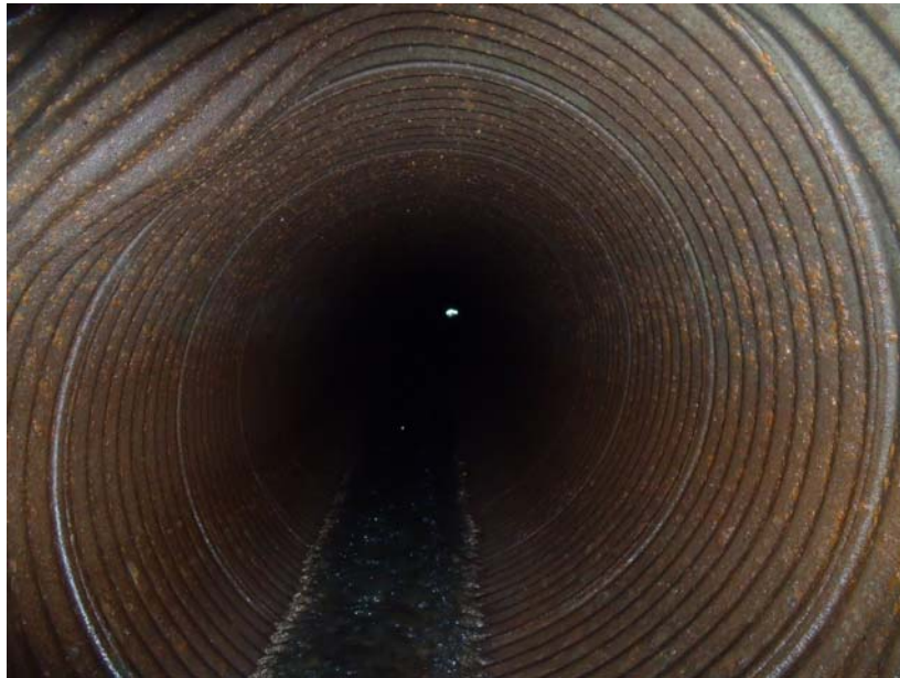
Figure 8: Deformed sewer at Joint – looking downstream
