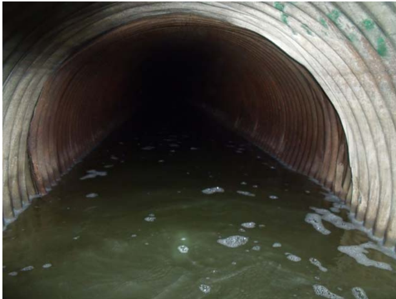
Figure 2: Reverse grade on pipe – looking down-stream
