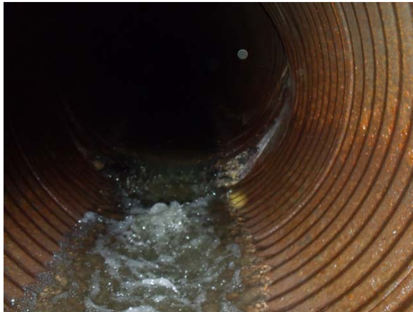
Figure 4: Large Displaced Joint (Probable location of sink hole) looking upstream
