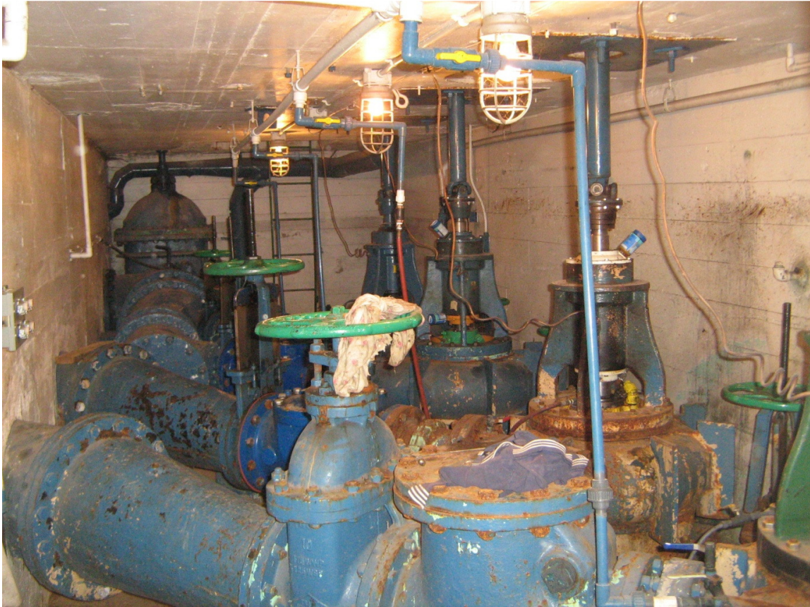
Figure 14 : Montcalm Pumping Station Pump Room
