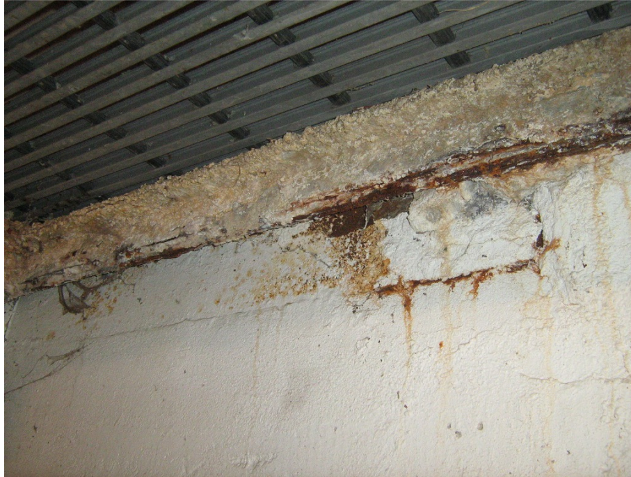
Figure 9 : Pump Room Ceiling Hatch
