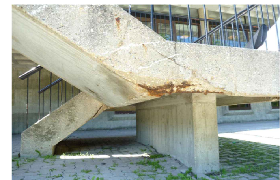
PHOTO #4: CRACKING AND DELAMINATION OF STAIR STRINGER.
