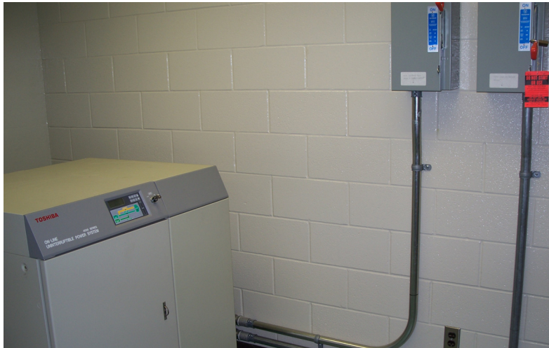
Figure 20.20: UPS - Not working as of August 2008
