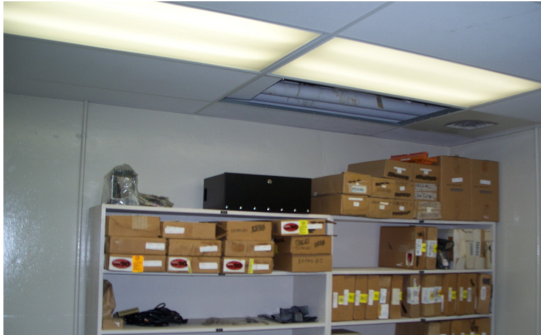
Figure 20.23: Computer Supplies Storage - Past Ceiling Leak
