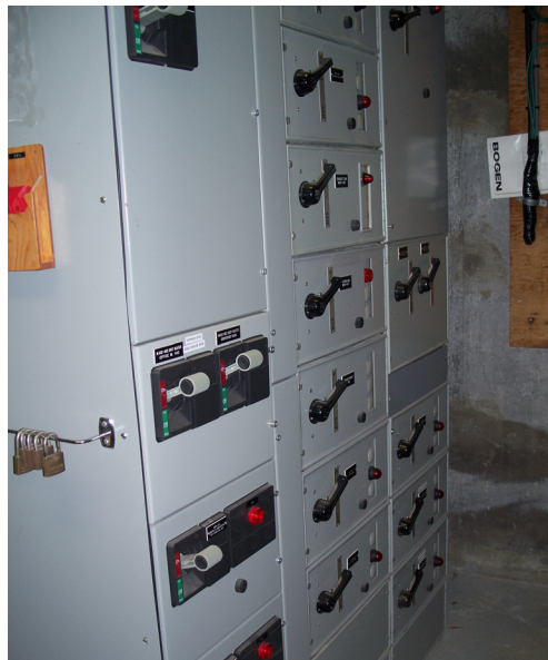
Figure 20.21: MCC-1M in the Admin Building Electrical Room
