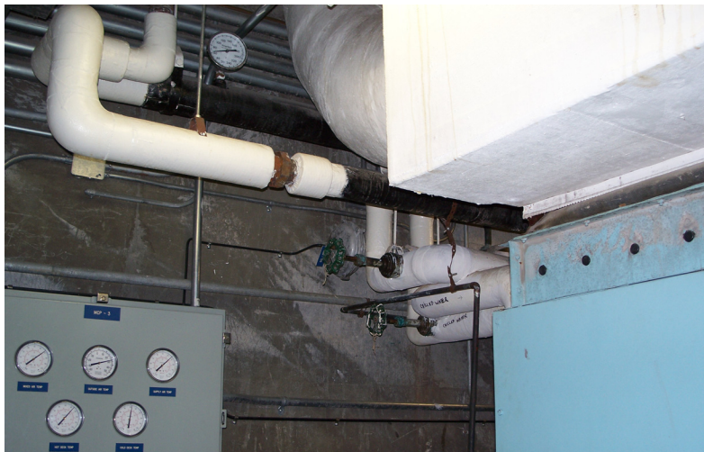
Figure 20.19: Air Handling Heat Exchanger and Piping
