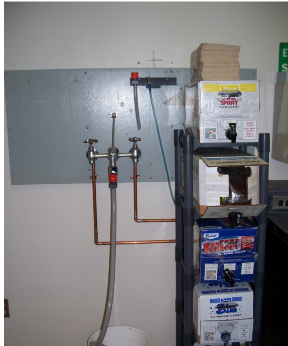
Figure 20.12: Room Fixtures and Laboratory Room Cleaners
