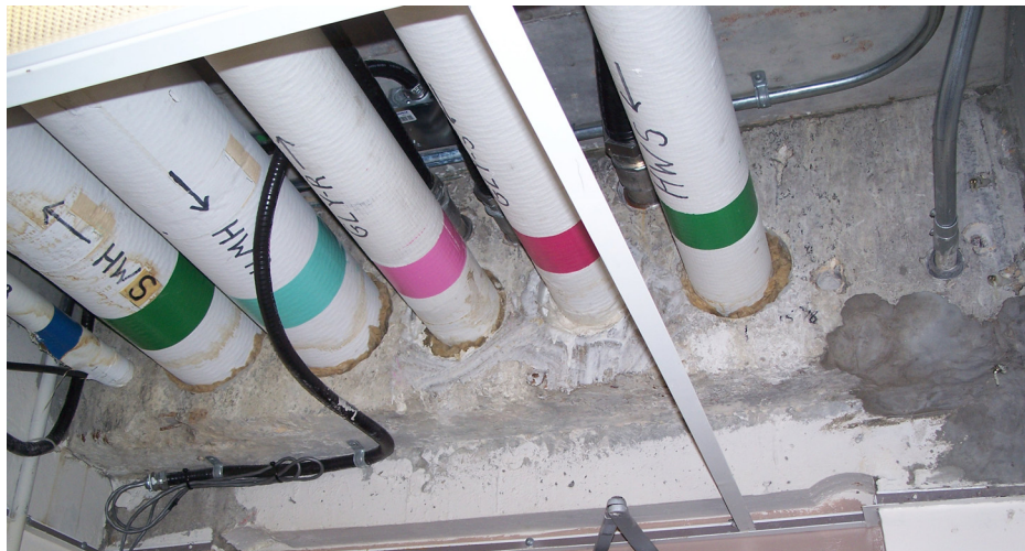
Figure 20.24: Leak Site at Corridor Portal
