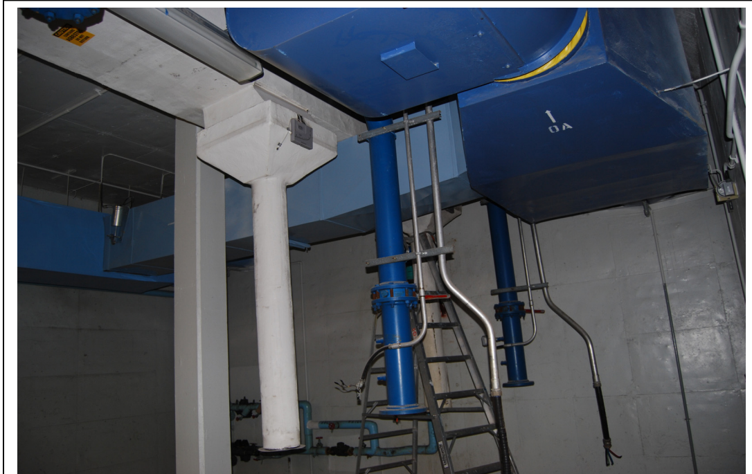
Figure 22.24: Water Service / Compressor Room facing east. Area ID #19.
