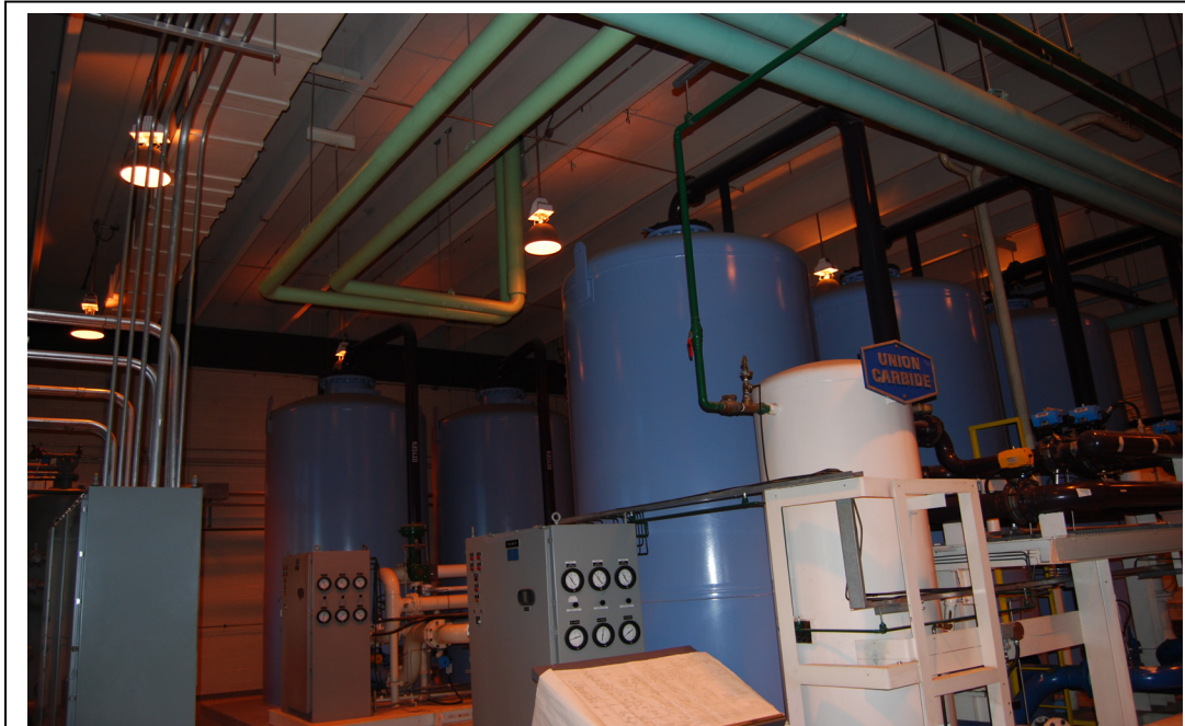
Figure 22.25: PSA / UNOX Equipment Room facing east. Area ID #20.
