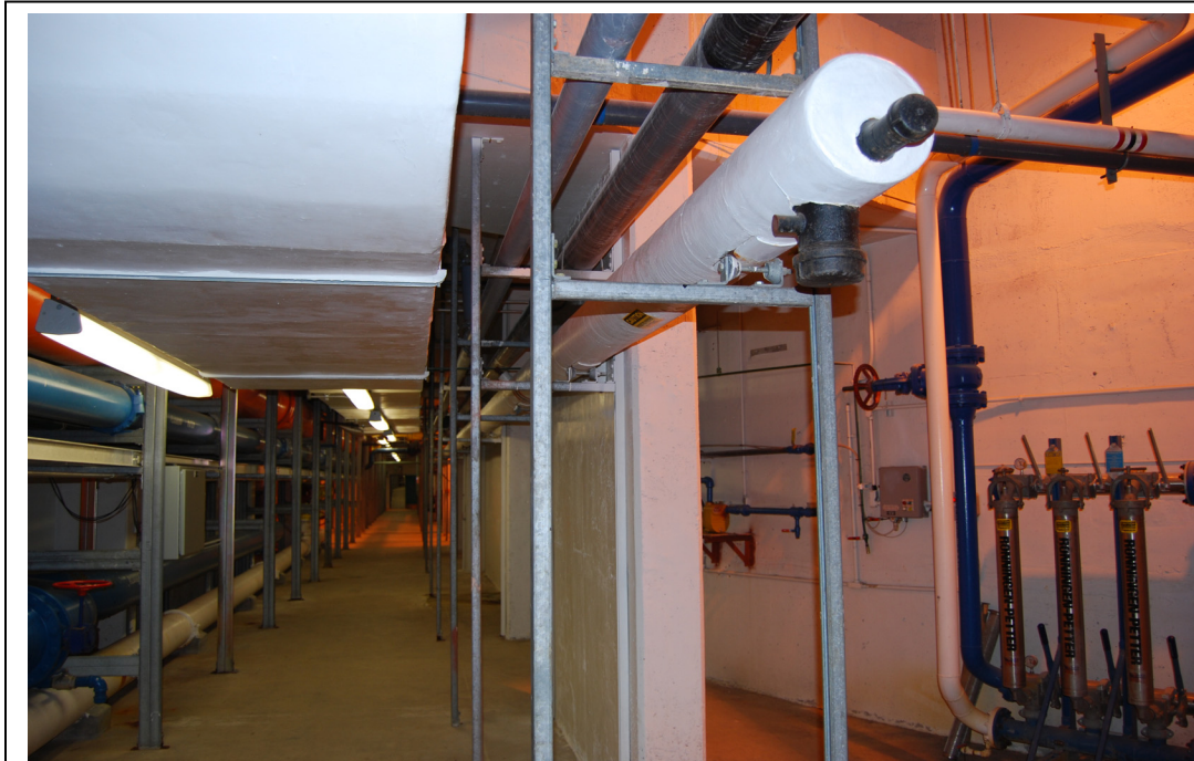
Figure 22.28: Gallery No. 3 facing east at end of Secondary Clarifier No. 1 & 2. Area ID #24/25.
