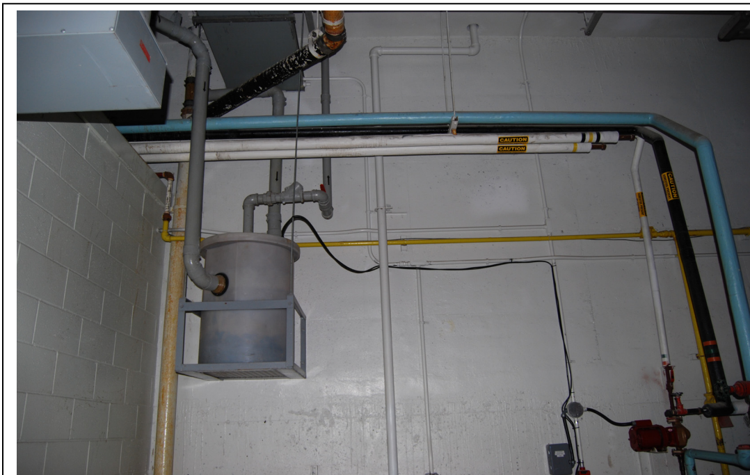
Figure 22.8: Boiler Room facing north. Area ID #11.
