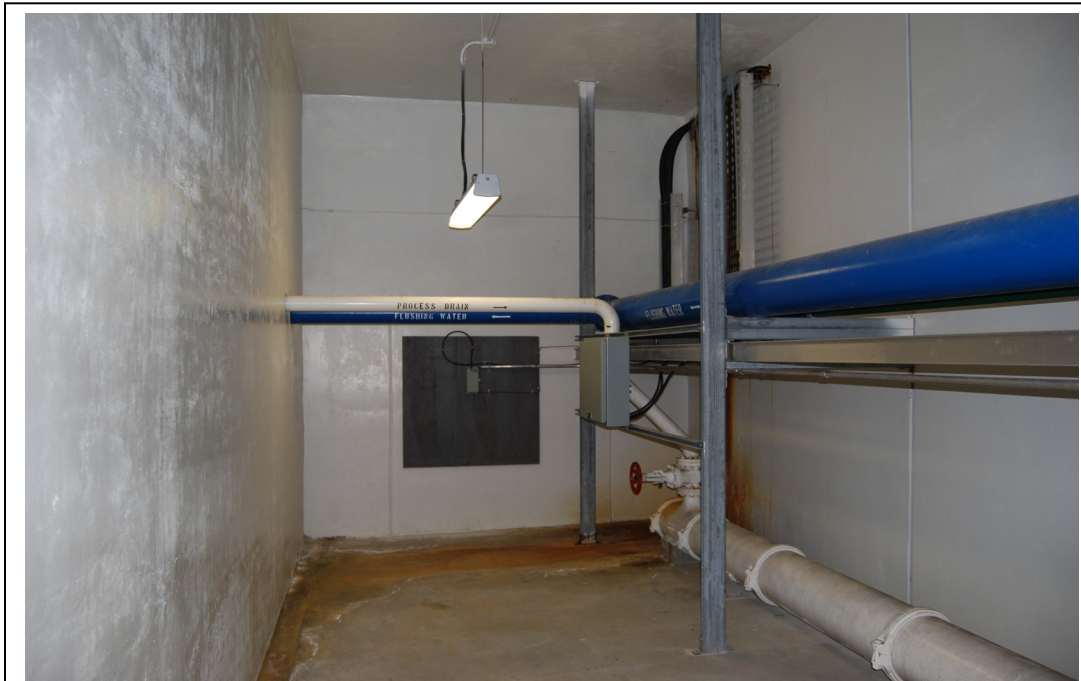
Figure 22.32: Gallery No. 3 facing west at end of Secondary Clarifier No. 3. Area ID #29.
