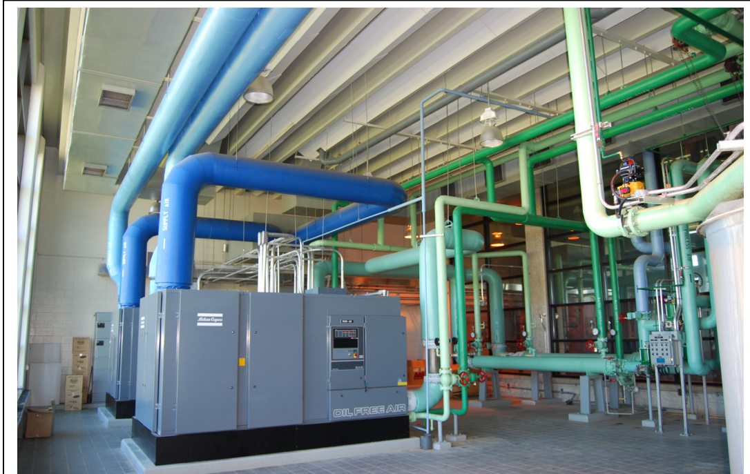
Figure 22.26: PSA Compressor Room facing east. Area ID #21.
