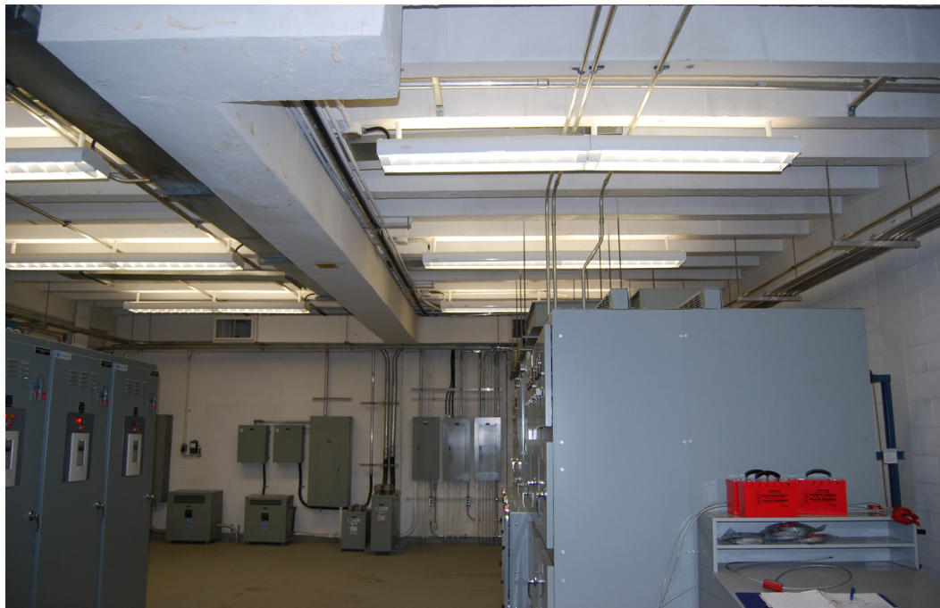
Figure 22.27: Electrical room east of Secondary Clarifier No. 1 facing north. Area ID #23.
