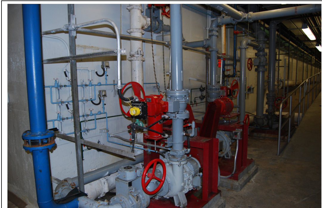
Figure 22.15: Gallery No. 3 at the Scum Pumping System for PST No. 1 & 2. Area ID #14.
