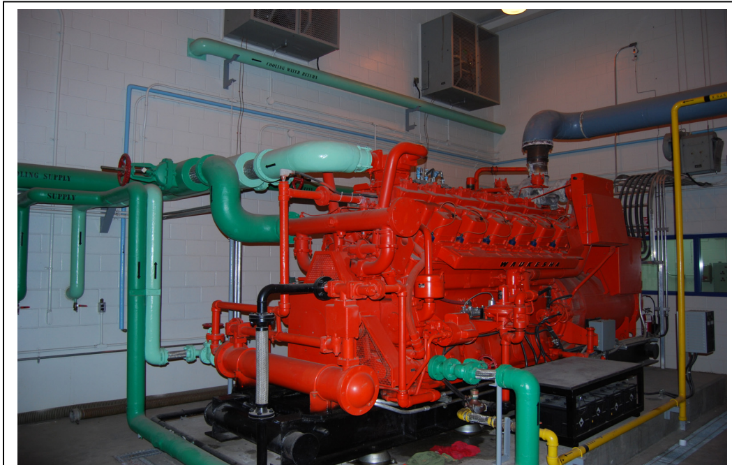
Figure 22.5: Standby power building generator. Area ID #9.
