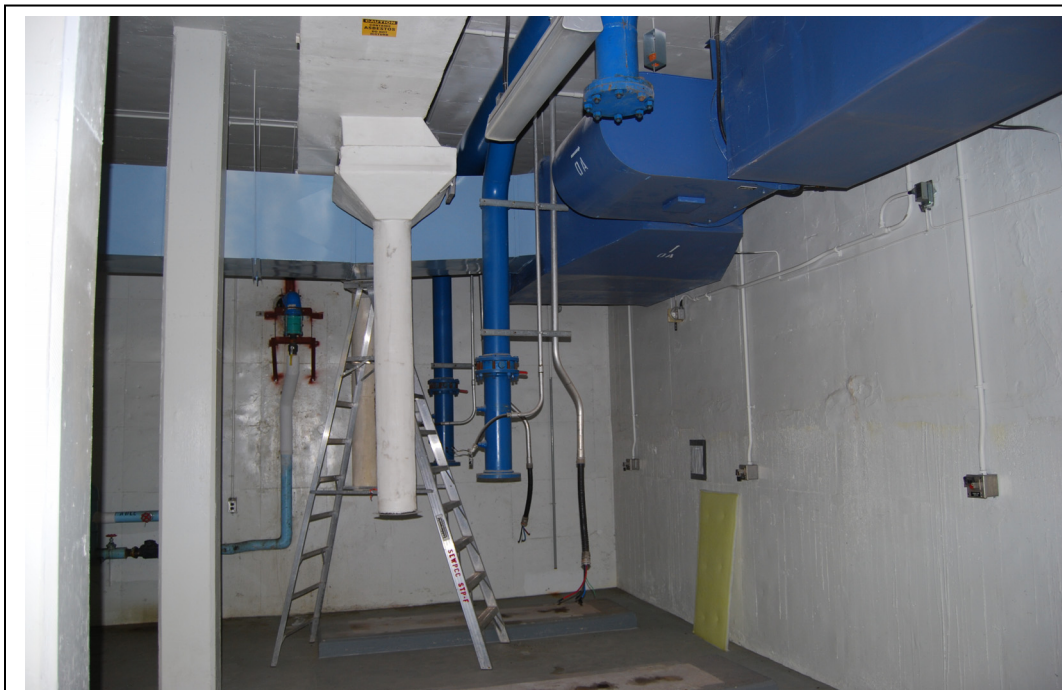
Figure 22.23: Water Service / Compressor Room facing east. Area ID #19.
