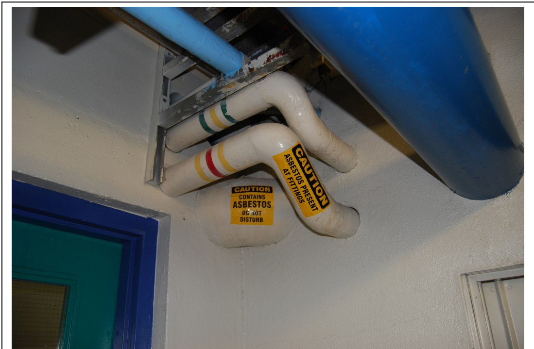
Figure 22.14: Gallery No. 3 east of entrance to Gallery No. 4 facing west. Area ID #14.
