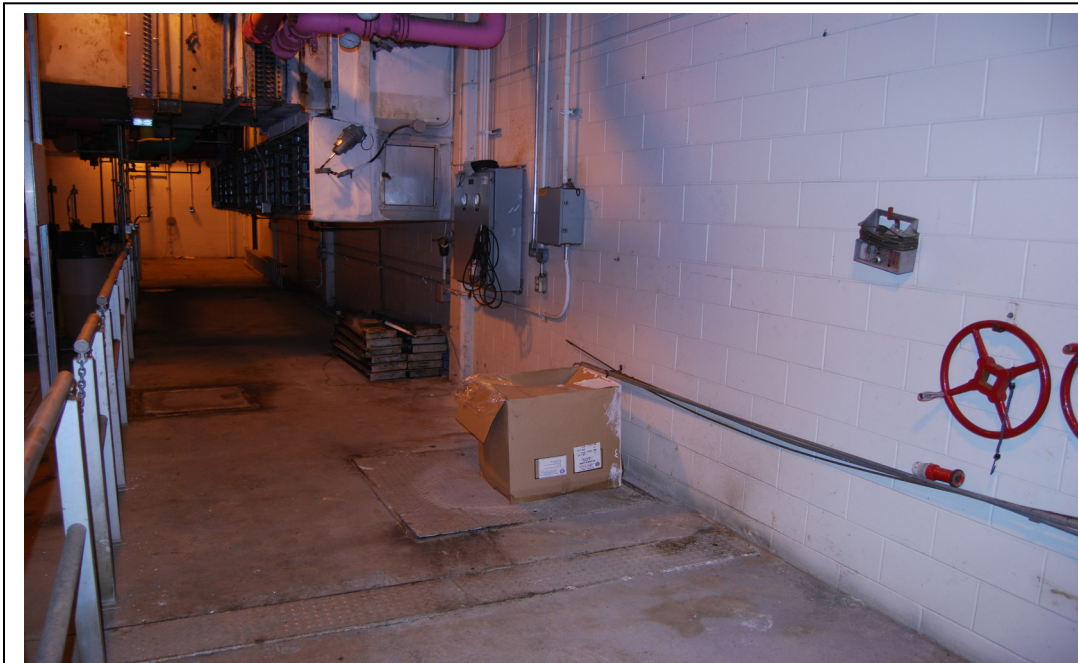
Figure 22.12: Influent end of PST No. 2 & 3 facing north. Area ID #13.
