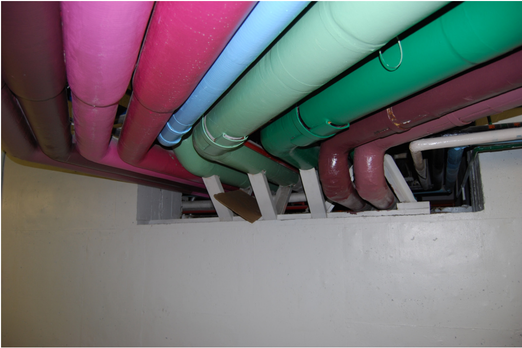
Figure 22.7: Gallery No. 3 at pipe chase to Boiler Room facing northeast. Area ID #11.
