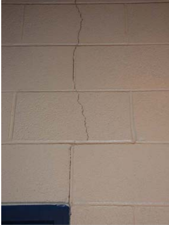
Photo 1.3- 35 – SECONDARY CLARIFIERS NOS. 1 AND 2 STRUCTURE Cracks in Concrete Block – Stairwell
