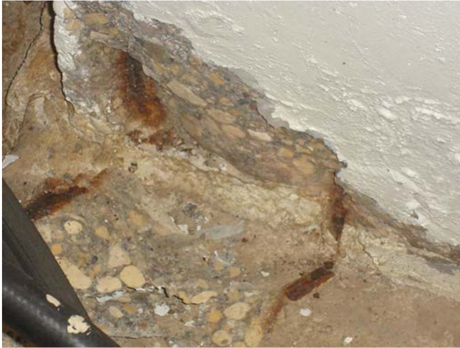
Photo 1.3-21 – PRIMARY CLARIFIER NOS. 1 AND 2 STRUCTURE Exposed Reinforcing Steel at Base of Concrete Tank This issue was addressed under Work Order 1005511, issued in 2010.
