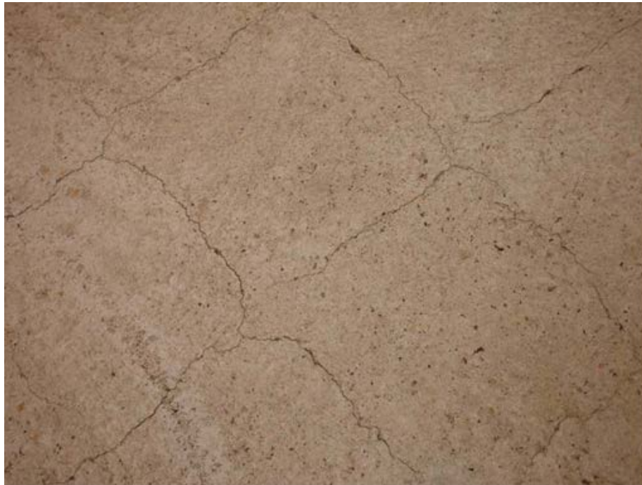
Photo 1.3-27 – SECONDARY CLARIFIER NO. 1 STRUCTURE Crack Pattern – Southwest Corner Clarifier No. 1 Walkway This issue has not been addressed since being noted in 2008.
