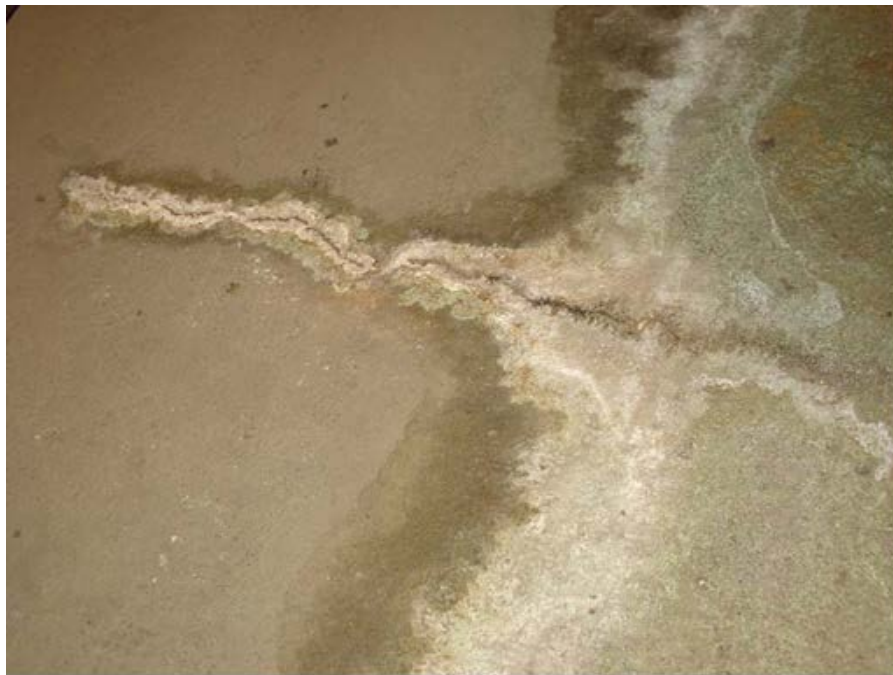
Photo 1.3-11 – GRIT BUILDING Efflorescence on Walkway Slab
