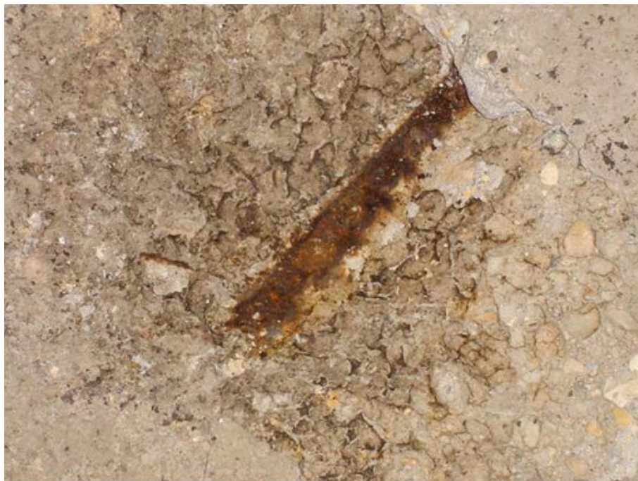
Photo 1.3-28 – SECONDARY CLARIFIER NO. 1 STRUCTURE Delaminated Concrete – Southwest Corner Clarifier No. 1 Walkway This issue has not been addressed since being noted in 2008.
