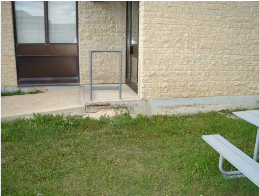
Photo 1.3-10 – PUMP AND SCREEN BUILDING Exposed Reinforcing Steel at Entry Slab This issue has not been addressed since being noted in 2008.
