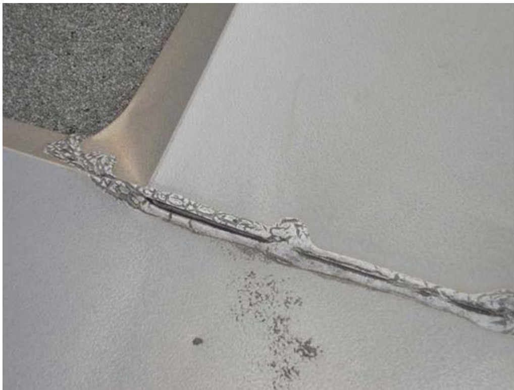
Photo 1.3-4 – ADMINISTRATION BUILDING AND EXPANSION Deterioration of Caulking at Parapet Flashing
