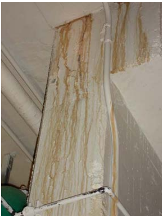
Photo 1.3-32 – SECONDARY CLARIFIER NOS. 1 AND 2 STRUCTURE Stained Concrete Column – Gallery No. 3 This issue has not been addressed since being noted in 2008.
