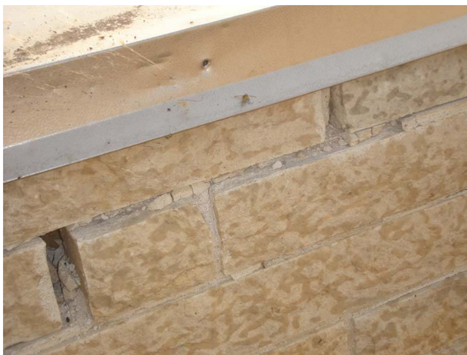
Photo 1.3-38 – SECONDARY CLARIFIERS NOS. 1 AND 2 STRUCTURE Loose Limestone Veneer in Upper Courses at Roof Parapet This issue has not been addressed since being noted in 2008.
