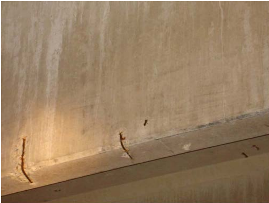
Photo 1.3_30 – SECONDARY CLARIFIER NO. 2 STRUCTURE Fan Room – South End This issue has not been addressed since being noted in 2008.
