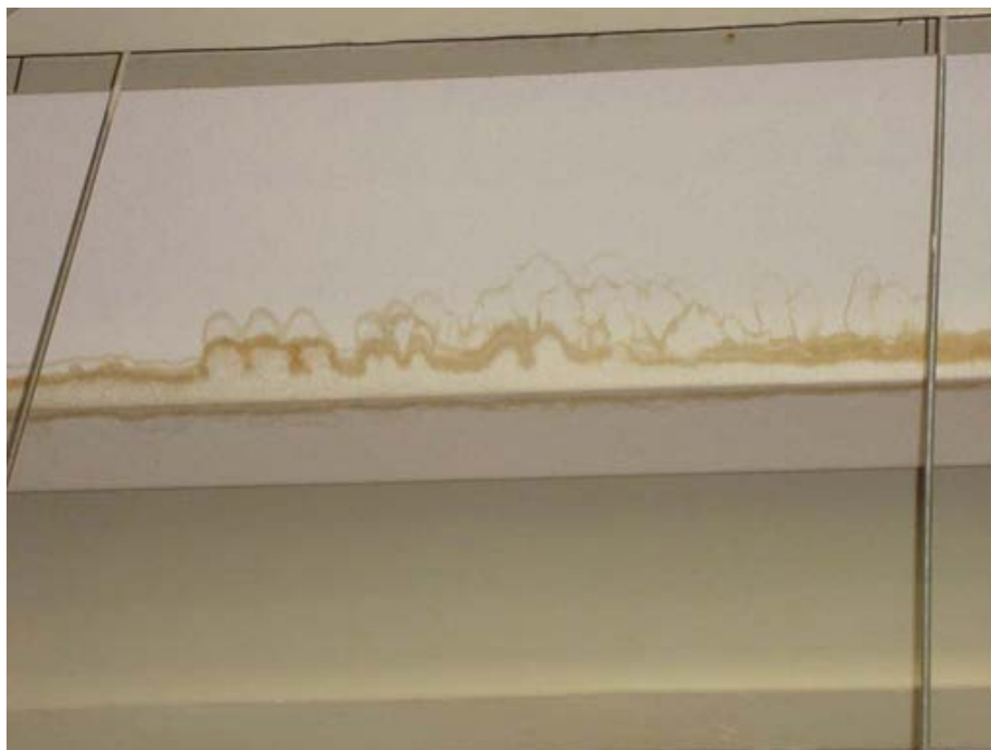
Photo 1.3-25 – PSA BUILDING Water Stained Acoustic Ceiling
