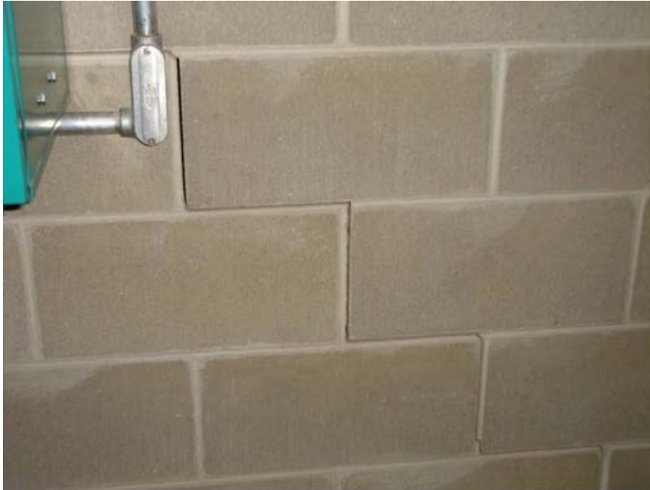
Photo 1.3-19 – MAINTENANCE/BOILER BUILDING “Ladder” cracks in Concrete Block Partition – Storage Room This issue has not been addressed since being noted in 2008.
