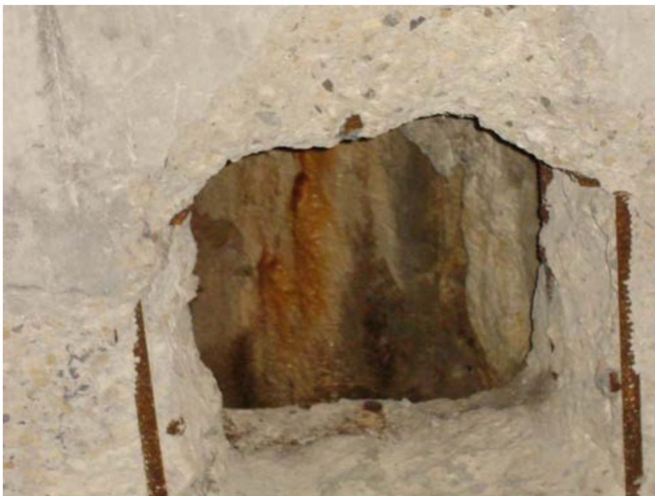
Photo 1.3-6 – PUMP AND SCREEN BUILDING Efflorescence on Ring Wall – Opening in Stairwell This issue has not been addressed since being noted in 2008.
