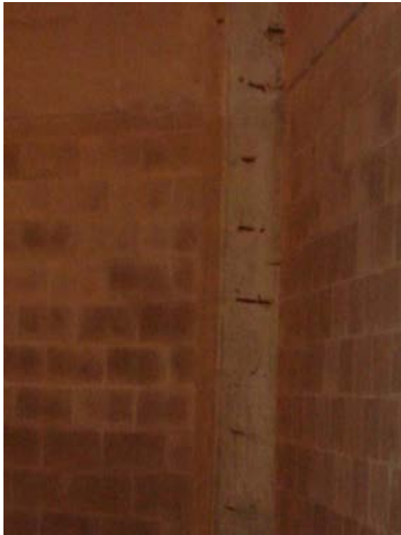
Photo 1.3-29 – SECONDARY CLARIFIER NO. 2 STRUCTURE Exposed Concrete Column Tiles – South End Clarifier No. 2 This issue has not been addressed since being noted in 2008.
