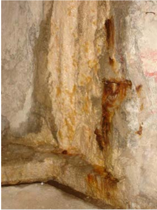
Photo 1.3-7 – PUMP AND SCREEN BUILDING Exposed Reinforcing Steel at base of Ring Wall – Dry Well This issue has not been addressed since being noted in 2008.
