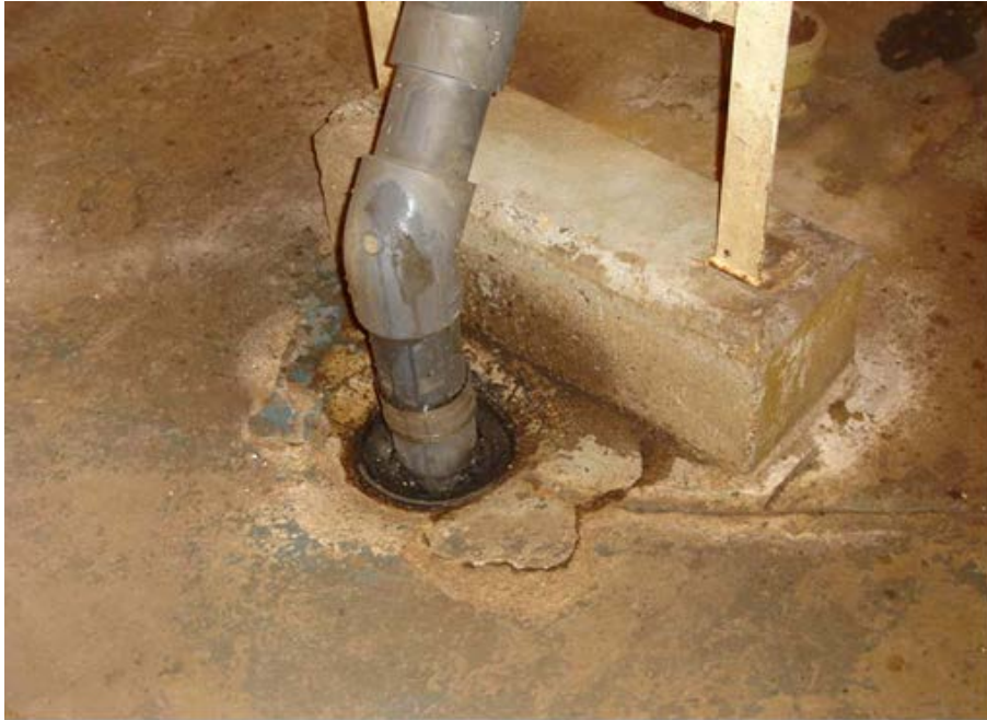
Photo 1.2-13 – GRIT BUILDING Spalled Concrete at Drain
