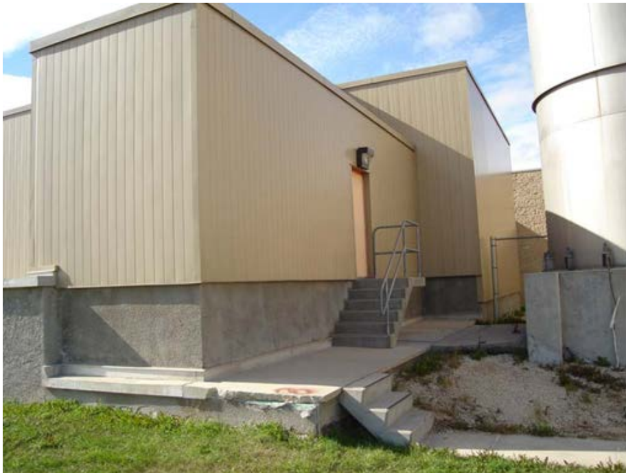
Photo 1.3-22 – PRIMARY CLARIFIER NO. 3 STRUCTURE Damaged Concrete – Entry Slab South East Corner This issue has not been addressed since being noted in 2008.
