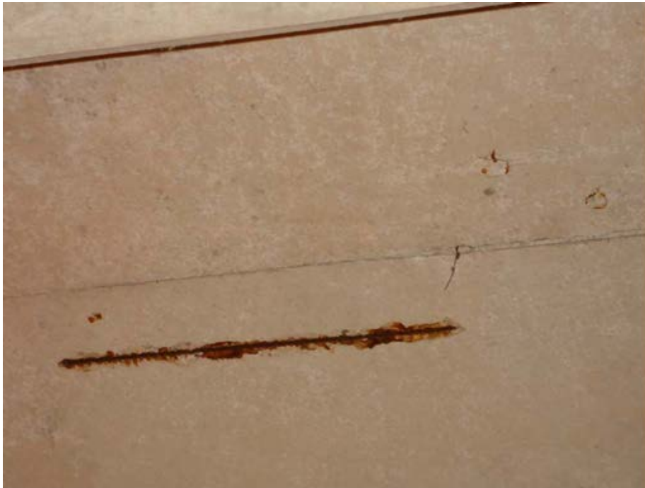
Photo 1.3-31 – SECONDARY CLARIFIER NO. 2 STRUCTURE Exposed Reinforcing Steel – Precast Roof Section – South End This issue has not been addressed since being noted in 2008.
