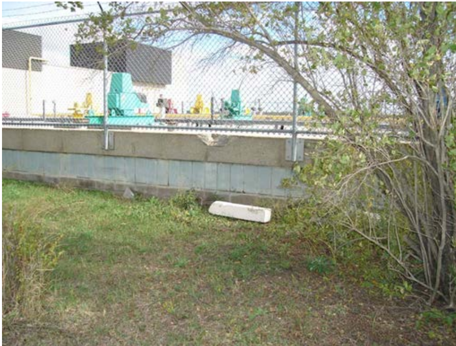
Photo 1.3-23 – OXYGEN REACTORS NOS. 1 AND 2 STRUCTURE Damaged Parapet – North Face
