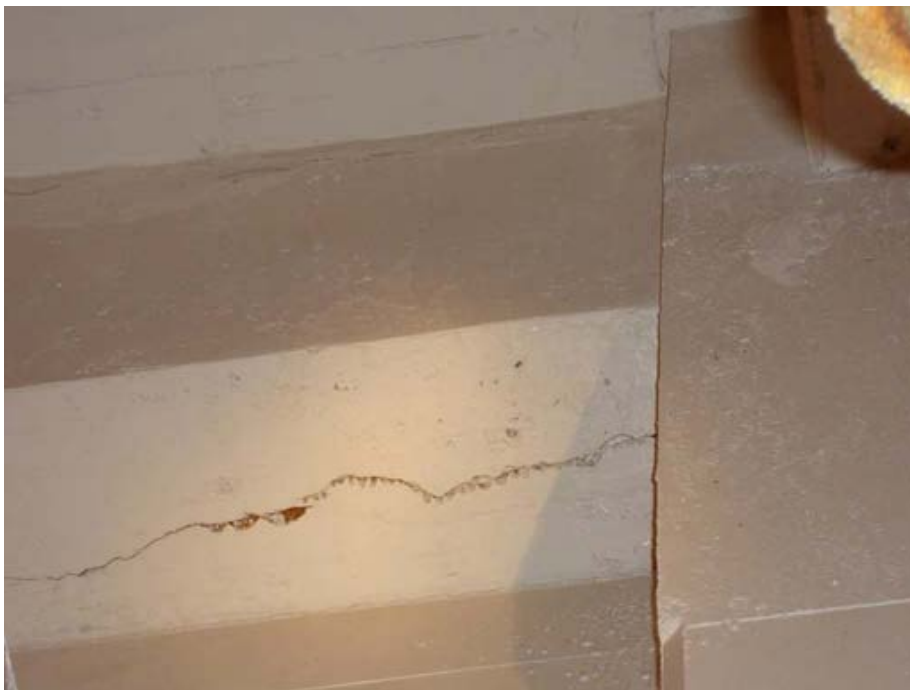
Photo 1.3-34 – SECONDARY CLARIFIER NOS. 1 AND 2 STRUCTURE Crack Along Underside of Beam – Gallery No. 3 This issue has not been addressed since being noted in 2008.
