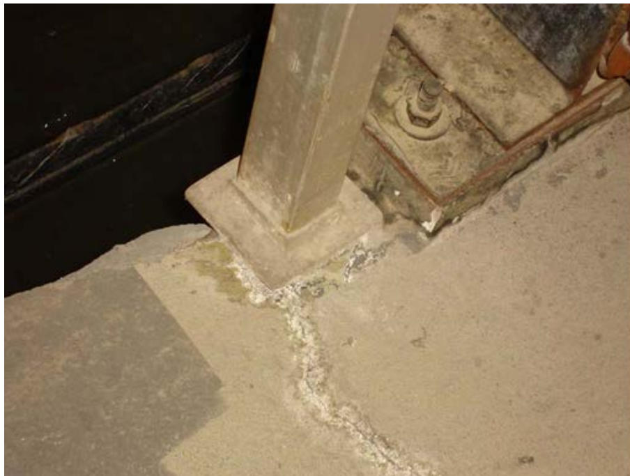
Photo 1.3-12 – GRIT BUILDING Spalled Concrete at Guardrail in Screen Room
