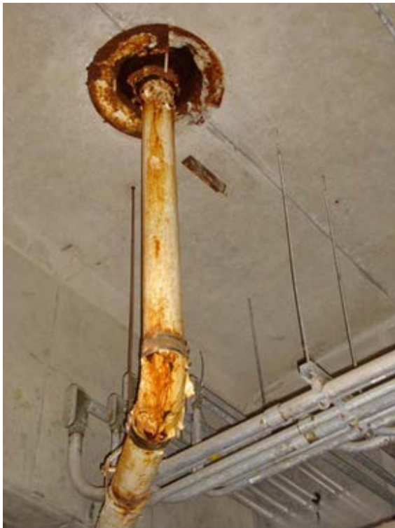
Photo 1.3-36 – SECONDARY CLARIFIER NOS. 1 AND 2 STRUCTURE Corrosion at Roof Drain
