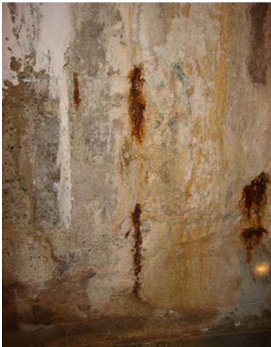
Photo 1.3-8 – PUMP AND SCREEN BUILDING Exposed Reinforcing Steel at Base of Ring Wall – Dry Well This issue has not been addressed since being noted in 2008.
