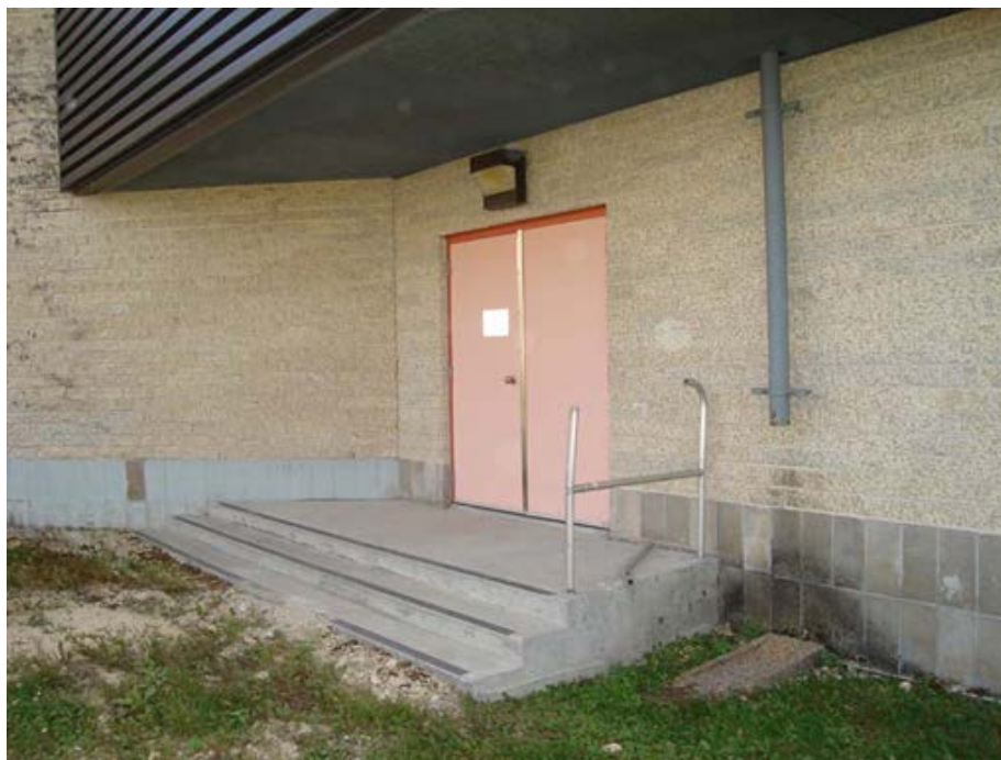
Photo 1.3-37 – SECONDARY CLARIFIERS NO. 1 STRUCTURE Broken Handrail – North Entrance noted in 2008. The handrail has been replaced.
