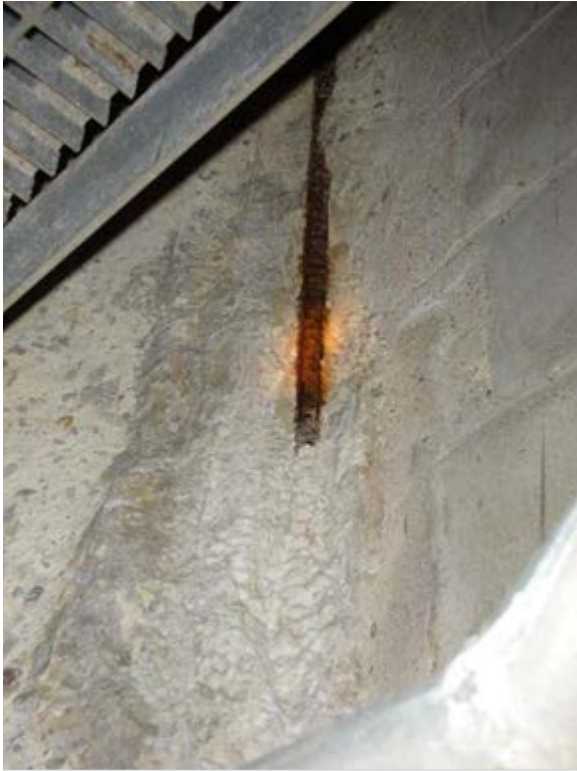
Photo 1.3-9 – PUMP AND SCREEN BUILDING Exposed Reinforcing Steel – Top of Dry Well This issue has not been addressed since being noted in 2008.
