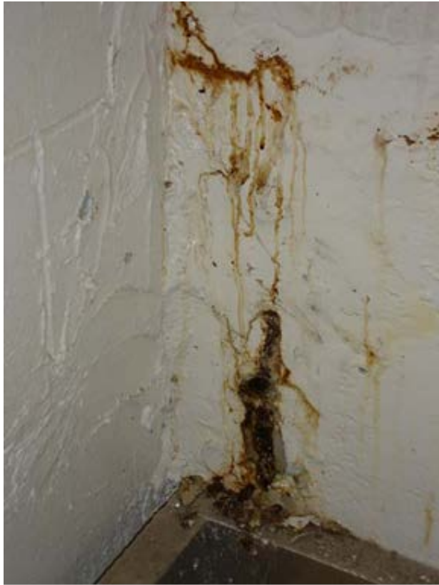
Photo 1.3-33 – SECONDARY CLARIFIER NOS. 1 AND 2 STRUCTURE Exposed Reinforcing Steel – Base of Concrete Tank Wall This issue has not been addressed since being noted in 2008.
