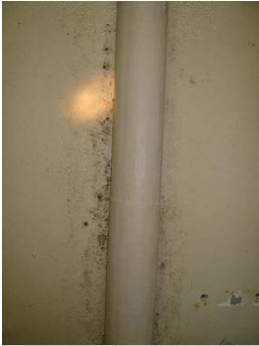
Photo 1.3-3 – ADMINISTRATION BUILDING EXPANSION Apparent Mould on Wall in Laboratory Storage Room noted in 2008.
