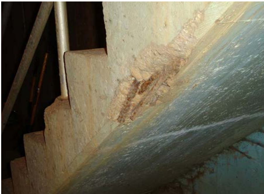
Photo 1.3-14 – GRIT BUILDING Exposed Reinforcing Steel at Concrete Stair in Grit Bin Area
