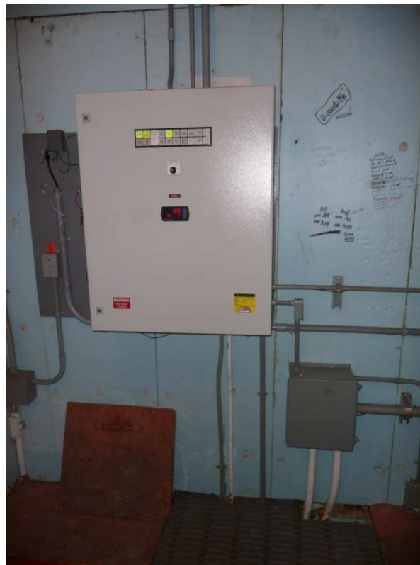
Figure 6-1 : Existing RTU Panel
