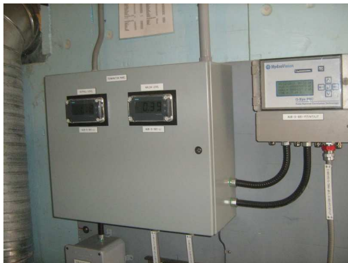
Figure 6-2 : Existing CSO Panel
