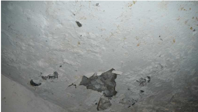
Figure 2-7 : Fluorescence on Ceiling of Pump Room
