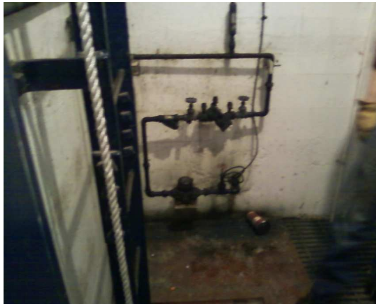
Figure 3-5 : Existing Water Service
