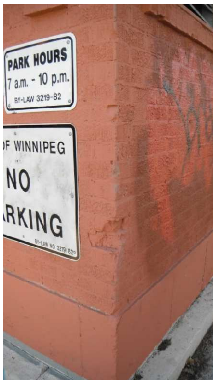
Figure 2-9 : Damaged Brick at Building Corner
