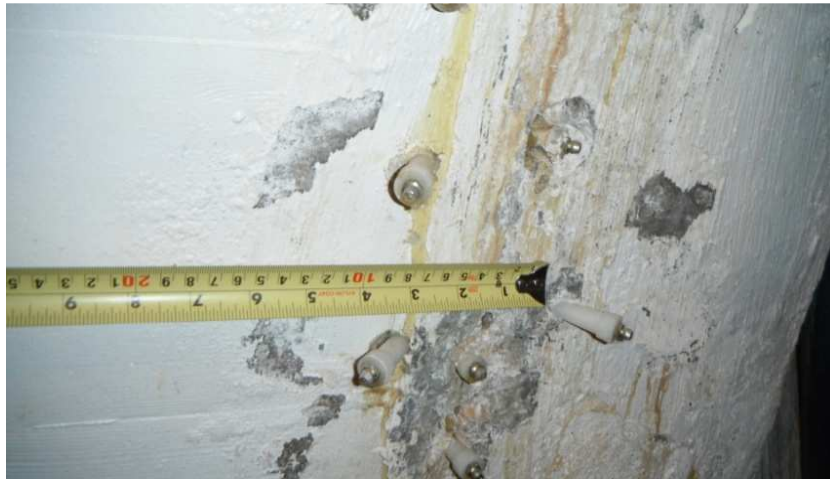
Figure 2-4 : Abandoned Epoxy Injection Ports in Motor Room
