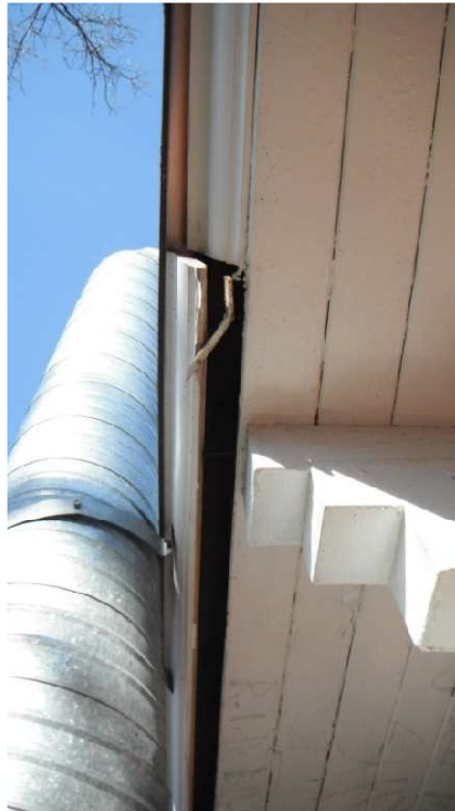
Figure 2-10 : Damaged Fascia Board
