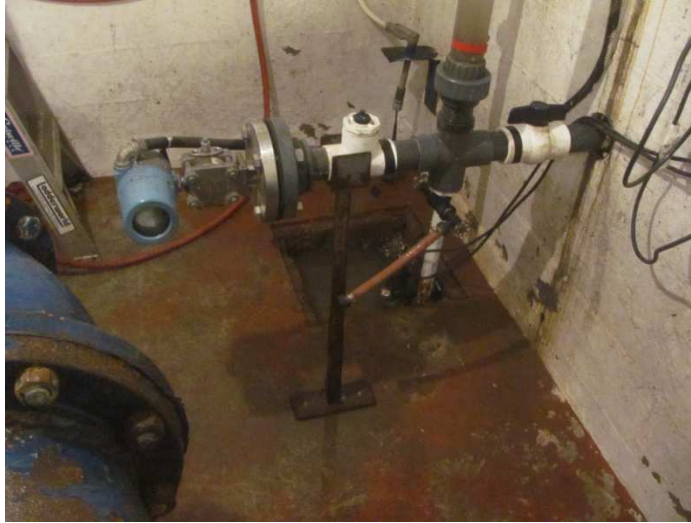
Figure 6-3 : Existing Level Sensor Installation
