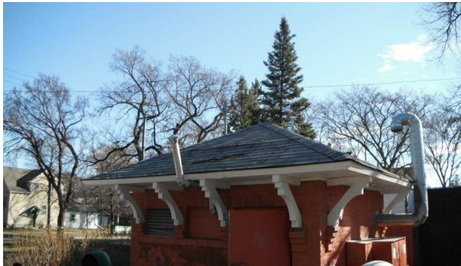
Figure 2-11 : Bulge in Roof
