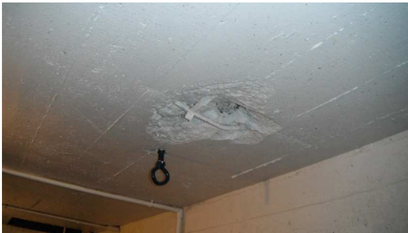
Figure 2-6 : Exposed Rebar in Ceiling of Pump Room
