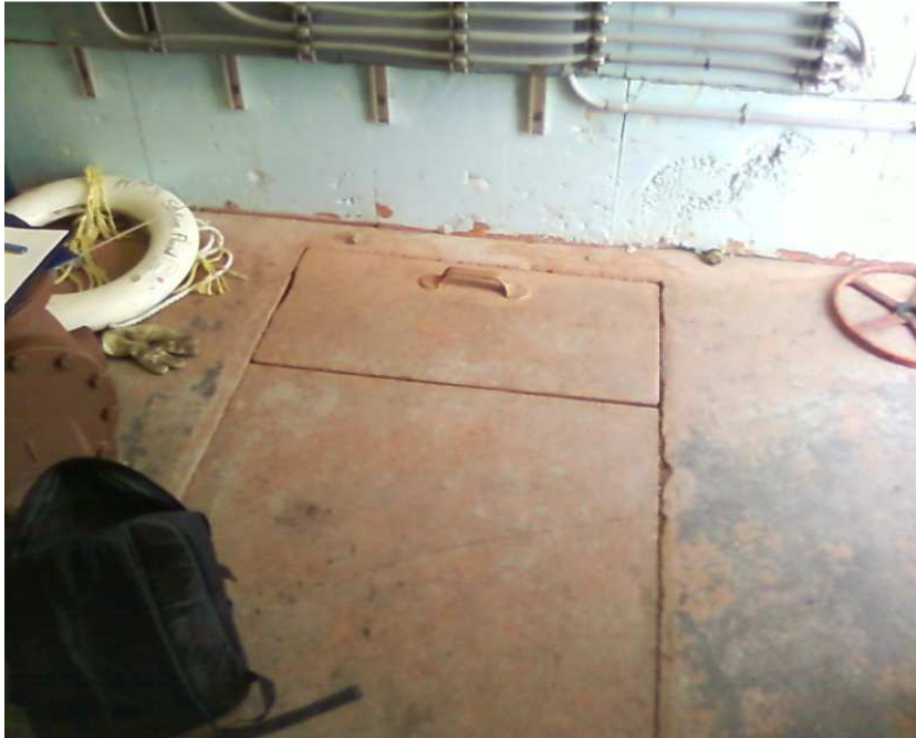
Figure 2-1 : Comminutor Chamber Main Floor Access Hatch
