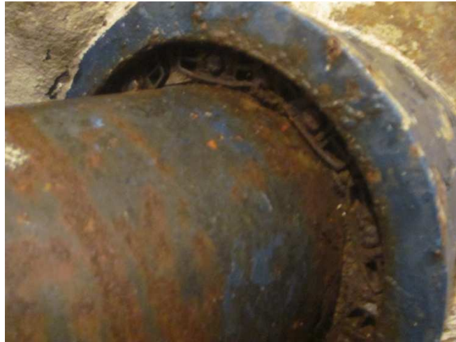
Figure 3-4 : Pump Suction Line
