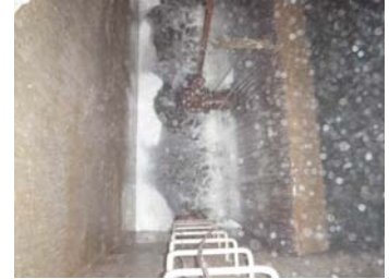
Typical City of Winnipeg chamber
