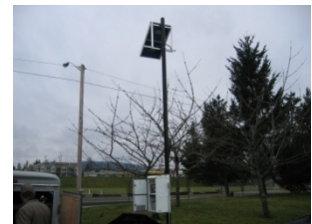
Pole mounted solar power system.
