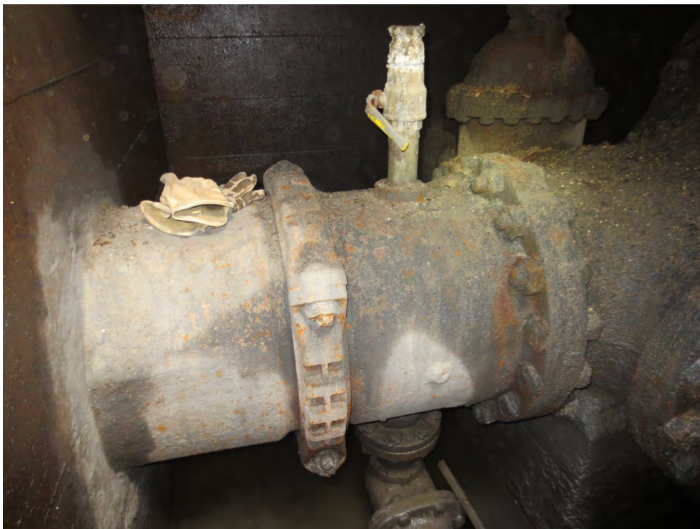
Figure 4 – Wilkes Ave Feedermain Offtake Chamber – Piping
