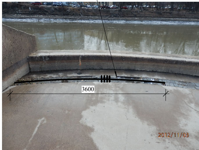
6 EXISTING PHOTO - MISSING PAVERS L4 Scale: 1:200
