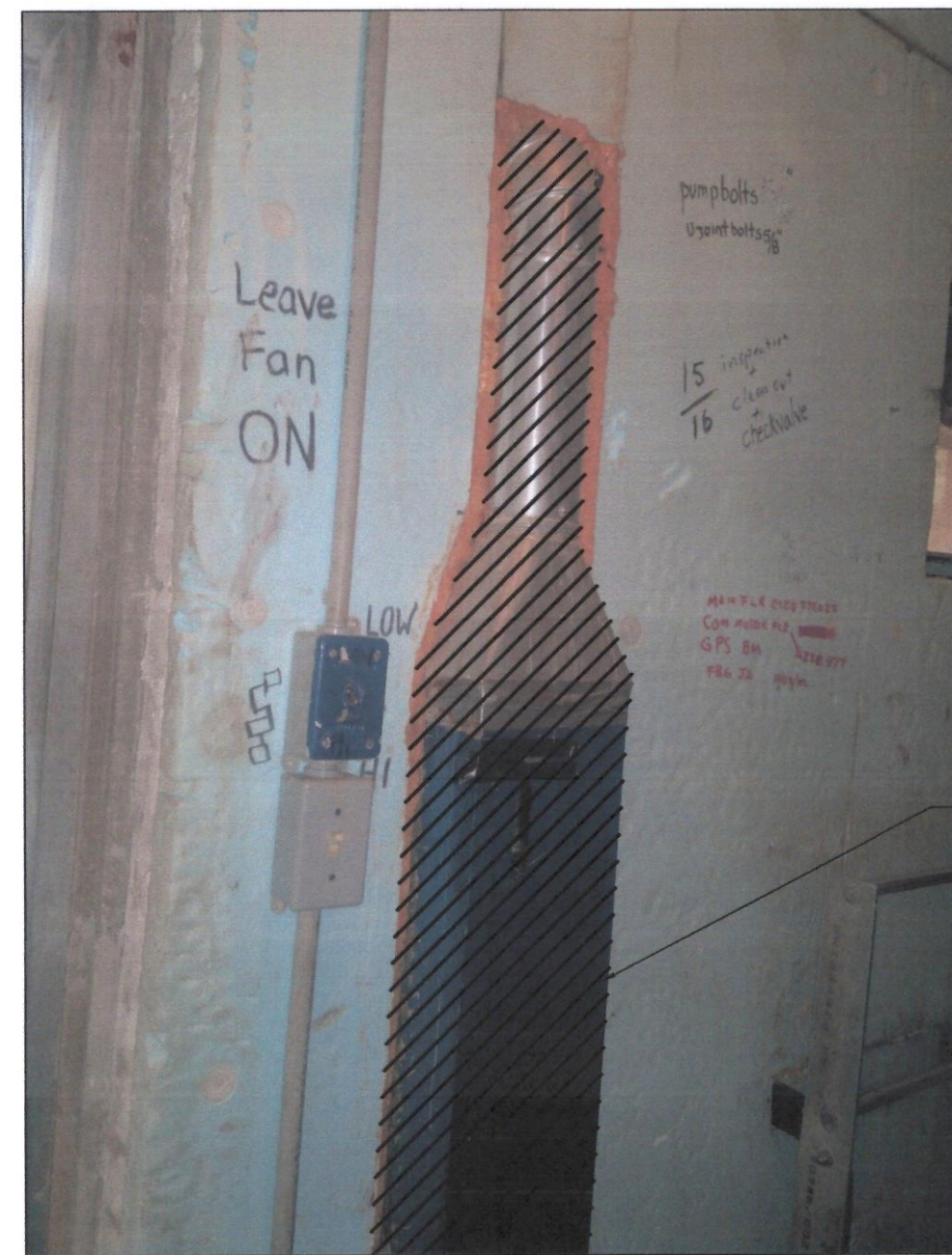
MAIN FLOOR – ELECTRICAL ROOM
