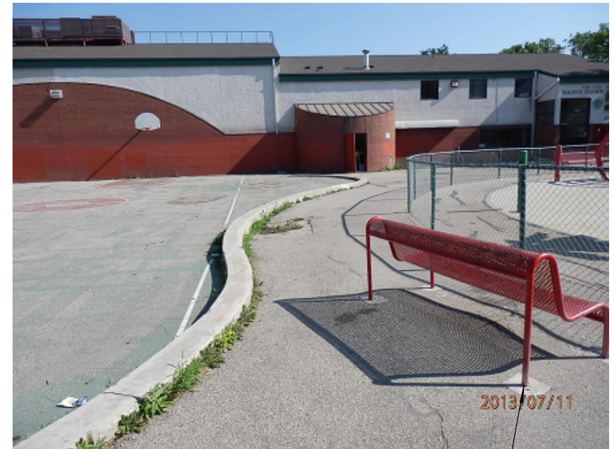
PHOTO "5": EXISTING BENCH TO BE REMOVED BY CUTTING METAL POST FLUSH WITH CONCRETE FOOTING, GRIND REMAINING METAL FOOTING LEVEL WITH CONCRETE FOOTING, AND FILL OLD METAL TUBE WITH MASONRY MORTAR.
