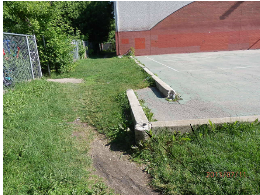
PHOTO "3": EXISTING CONCRETE CURB AND POST FOOTINGS TO BE REMOVED. POST FOOTINGS USE TO SUPPORT LOW CHAIN LINK FENCE. PULL CONCRETE FOOTING OUT OF THE GROUND AND FILL HOLE WITH COMPACTED SAND.
