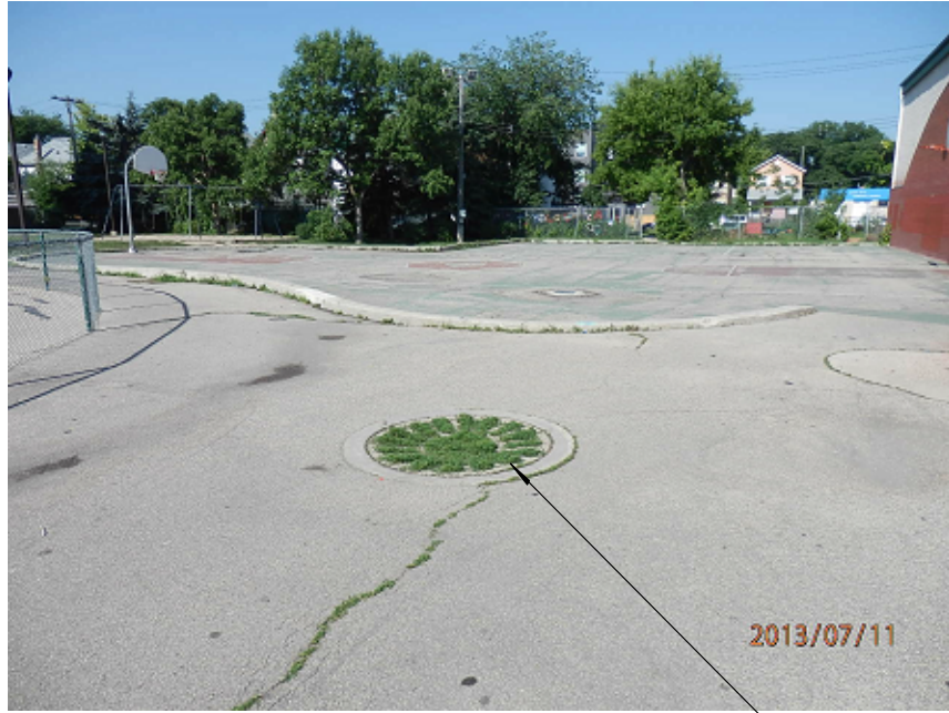
PHOTO "1": EXISTING CONCRETE TREE GRATE TO BE REMOVED AND FILLED IN WITH NEW CONCRETE PAVING
