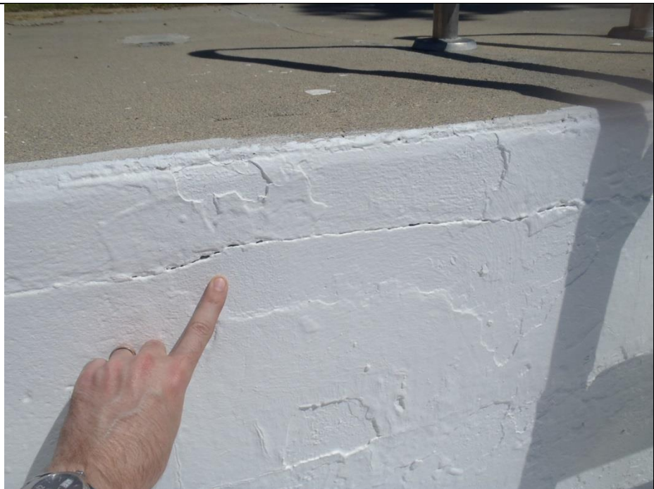
Photograph #2: Pour line separation between deck and pool wall.
