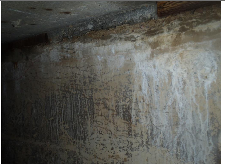
Photograph #4: Mechanical tunnel – pool wall – efflorescence and freeze/thaw cracking.
