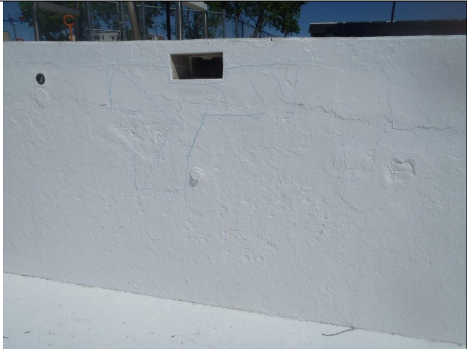
Photograph #1: Delaminated area (blue chalk outline) on pool wall.
