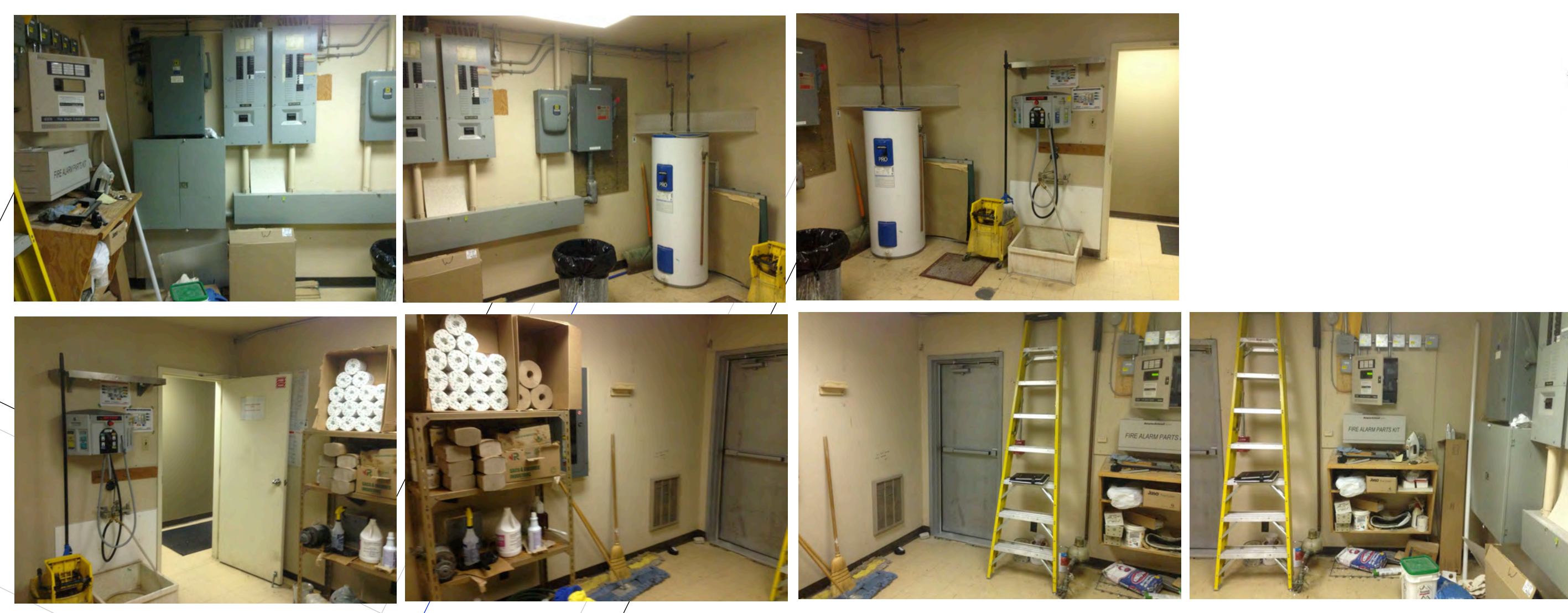
7 Mechanical Room At East End Cultural Centre L-2
