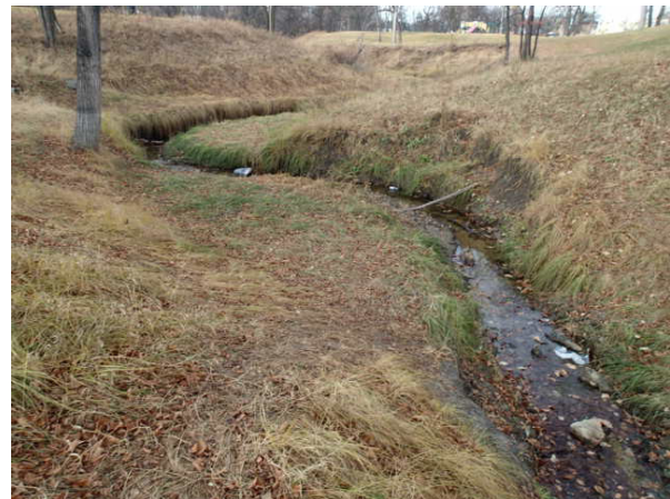
Figure 07 Toe Slump Upstream of Crossing
