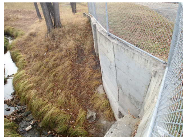
Figure 09 Bank at NW Wingwall
