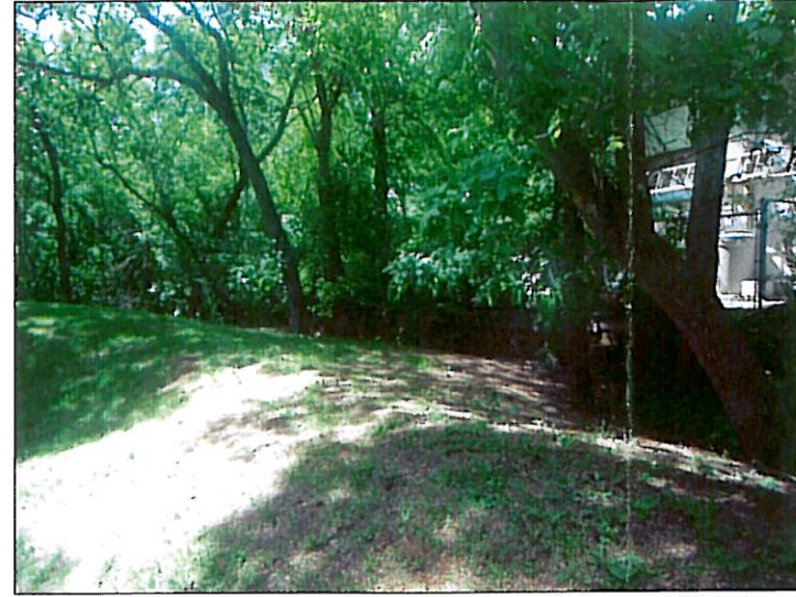
PHOTOGRAPH #2: FACING SOUTH SHOWING EXISTING RETAINING WALL AT NEIGHBOUR'S PROPERTY RELATIVE TO CLAY DYKE.
