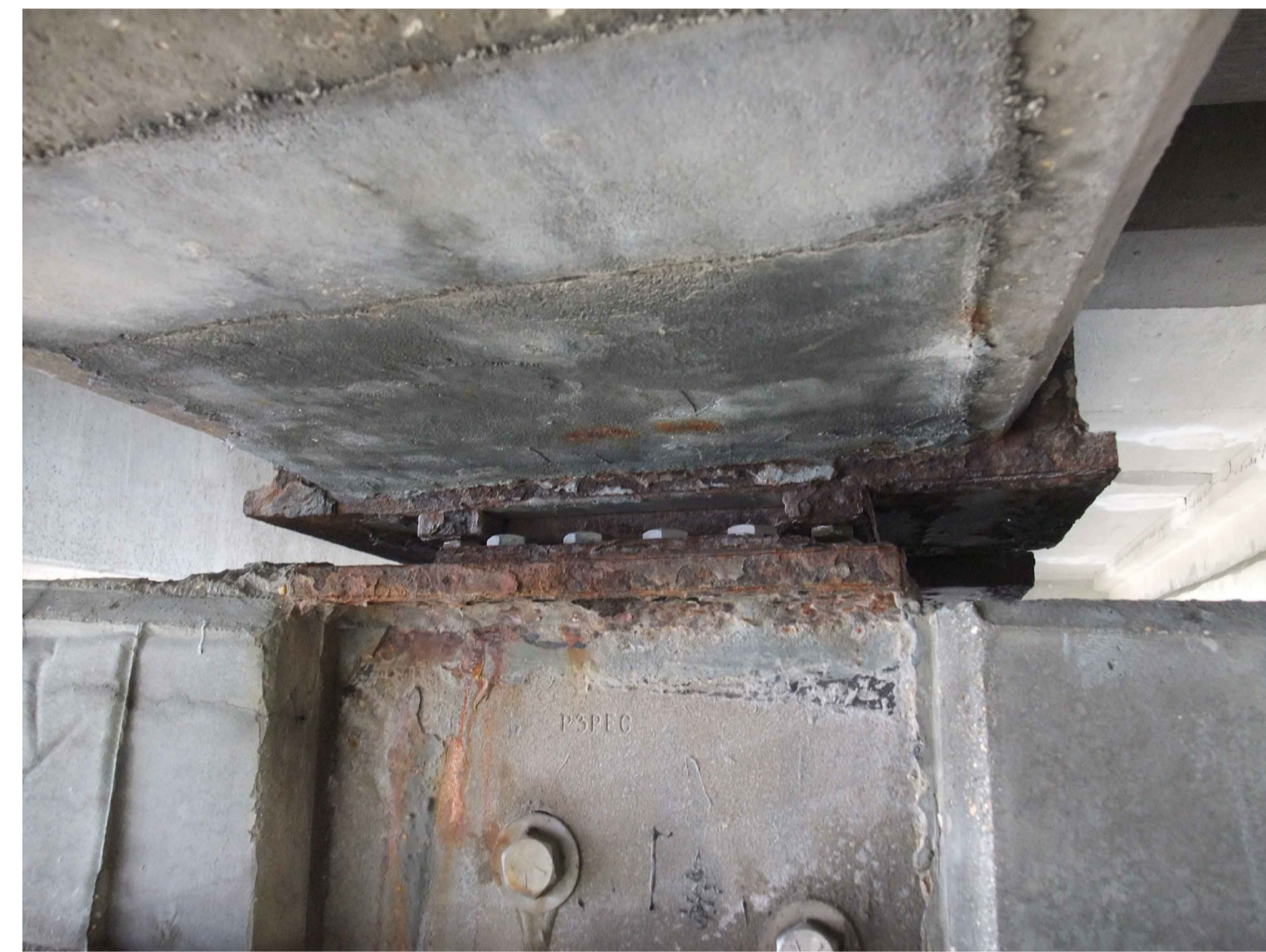
PHOTO - TYPICAL GUIDE BEARING EXISTING CONDITIONS
