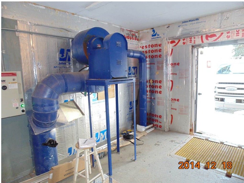
Photo 5 - Supply Fan Location in Main Floor Electrical Room
