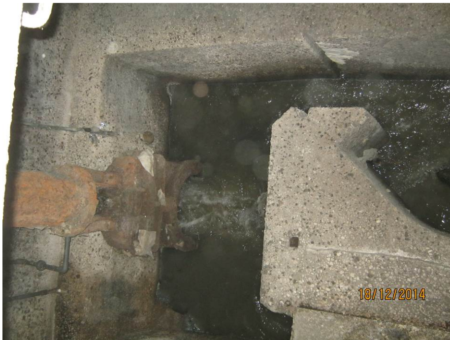
Photo 4 - 20" Comminutor Inlet Valve
