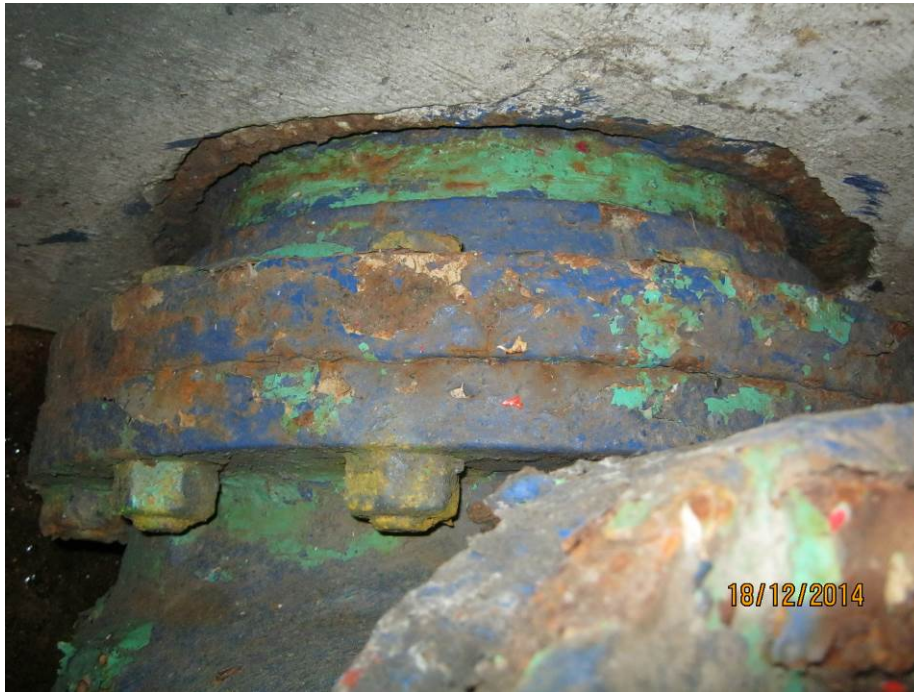
Photo 1 - Pump Suction Wall Insert
