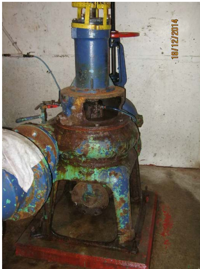
Photo 2 - One of Two Existing Pumps
