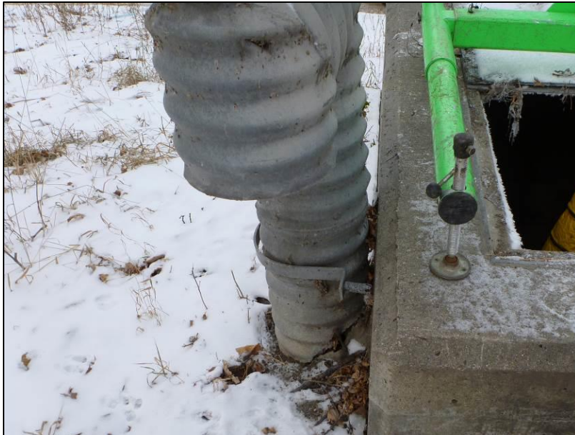
Photograph No. 3 Damage to air vent and anchor
