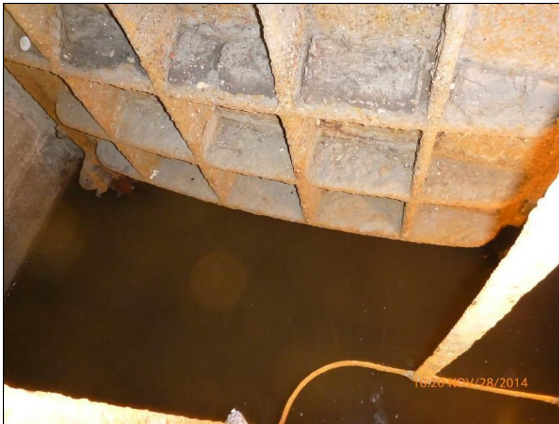
Photograph No. 9 Positive sluice gate
