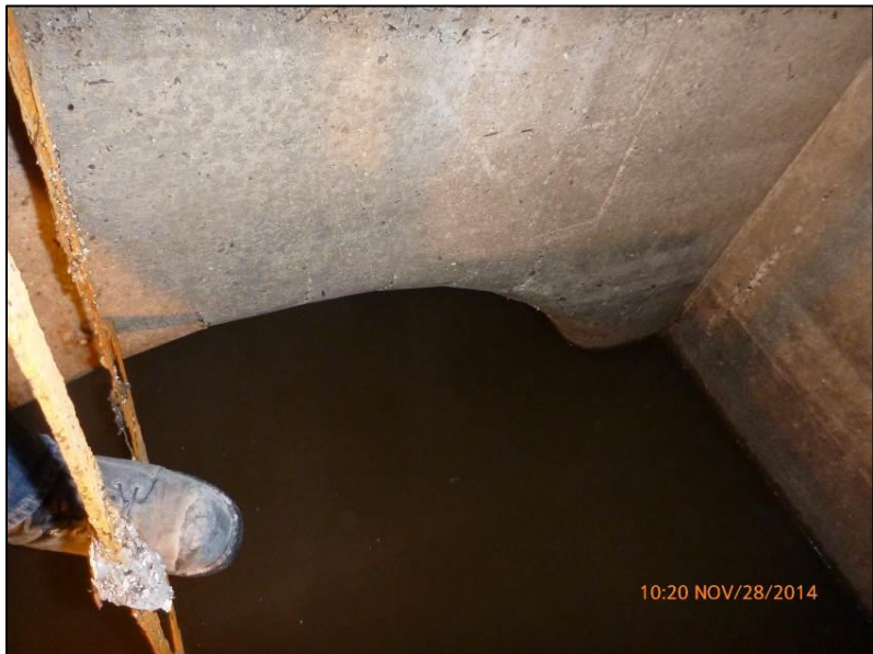
Photograph No. 4 Corrosion and section loss to ladder safety cage
