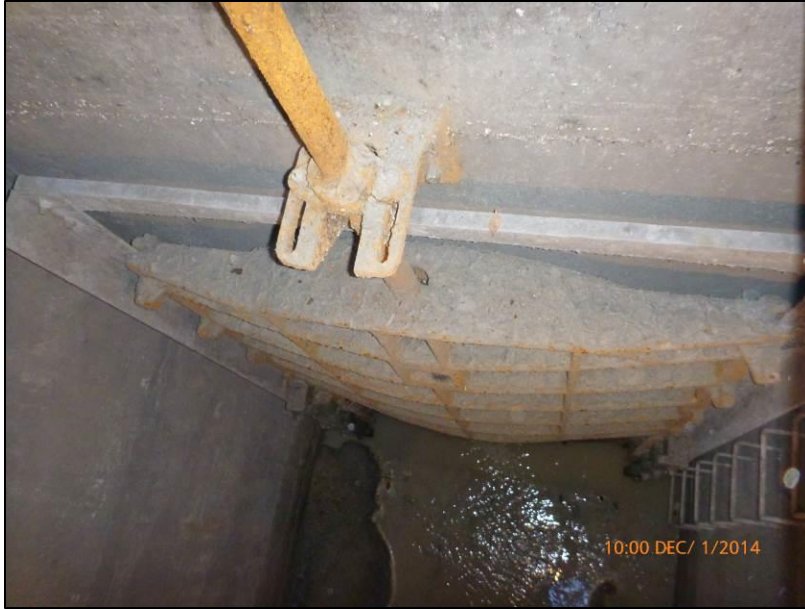
Photograph No. 9 Positive sluice gate
