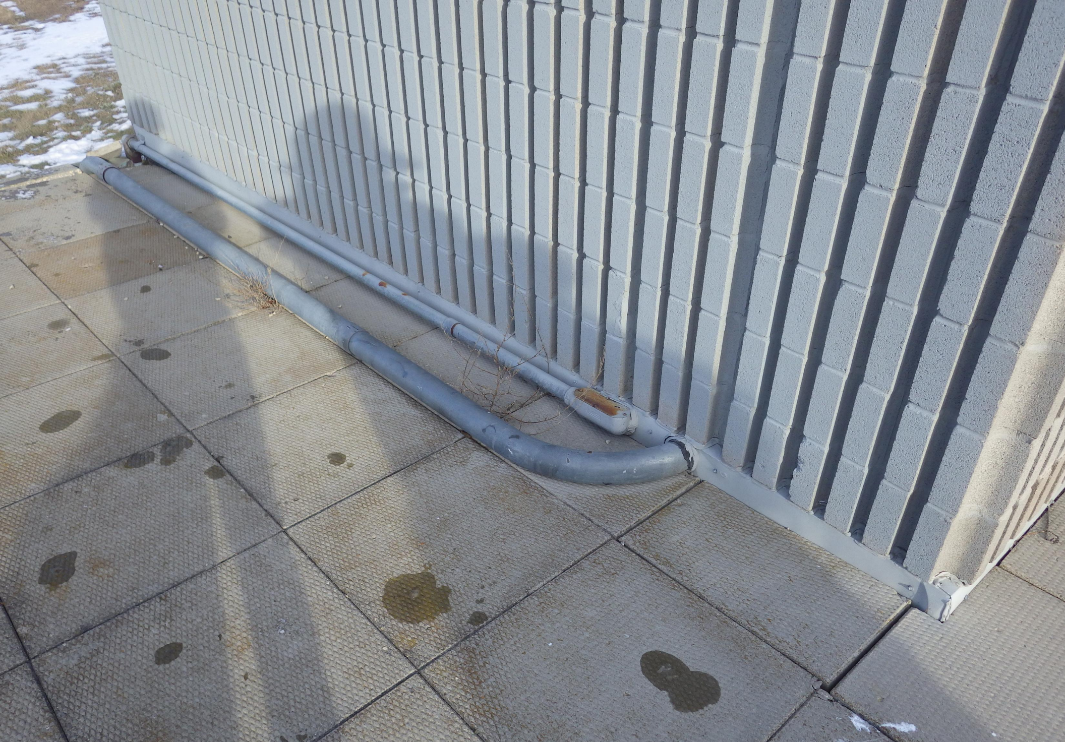
Access Building Electrical
