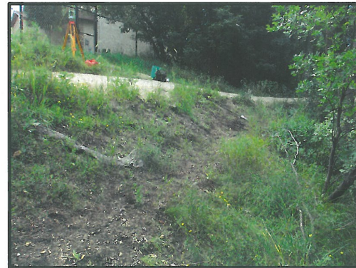
PHOTOGRAPH 5: FACING SOUTHEAST, SHOWING MID BANK AREA BETWEEN WALKWAY AND SHORELINE THAT WILL BE RE-GRADED. PROPOSED RETAINING WALL LOCATION WILL BE ALONG RIVERSIDE EXISTING EDGE OF WALKWAY.
