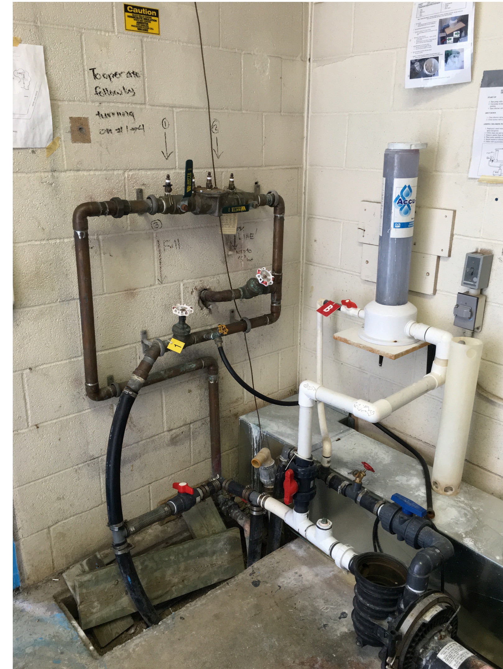
6 Existing Mechanical Room L-3
