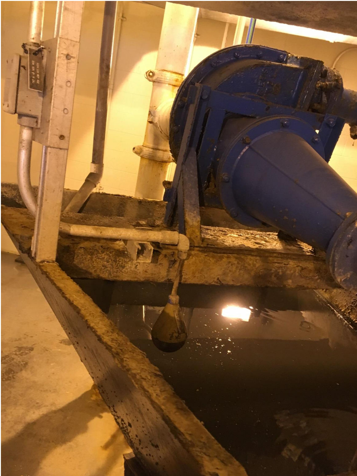
Figure 5: Grit Classifier H330 Float/Level Switch
