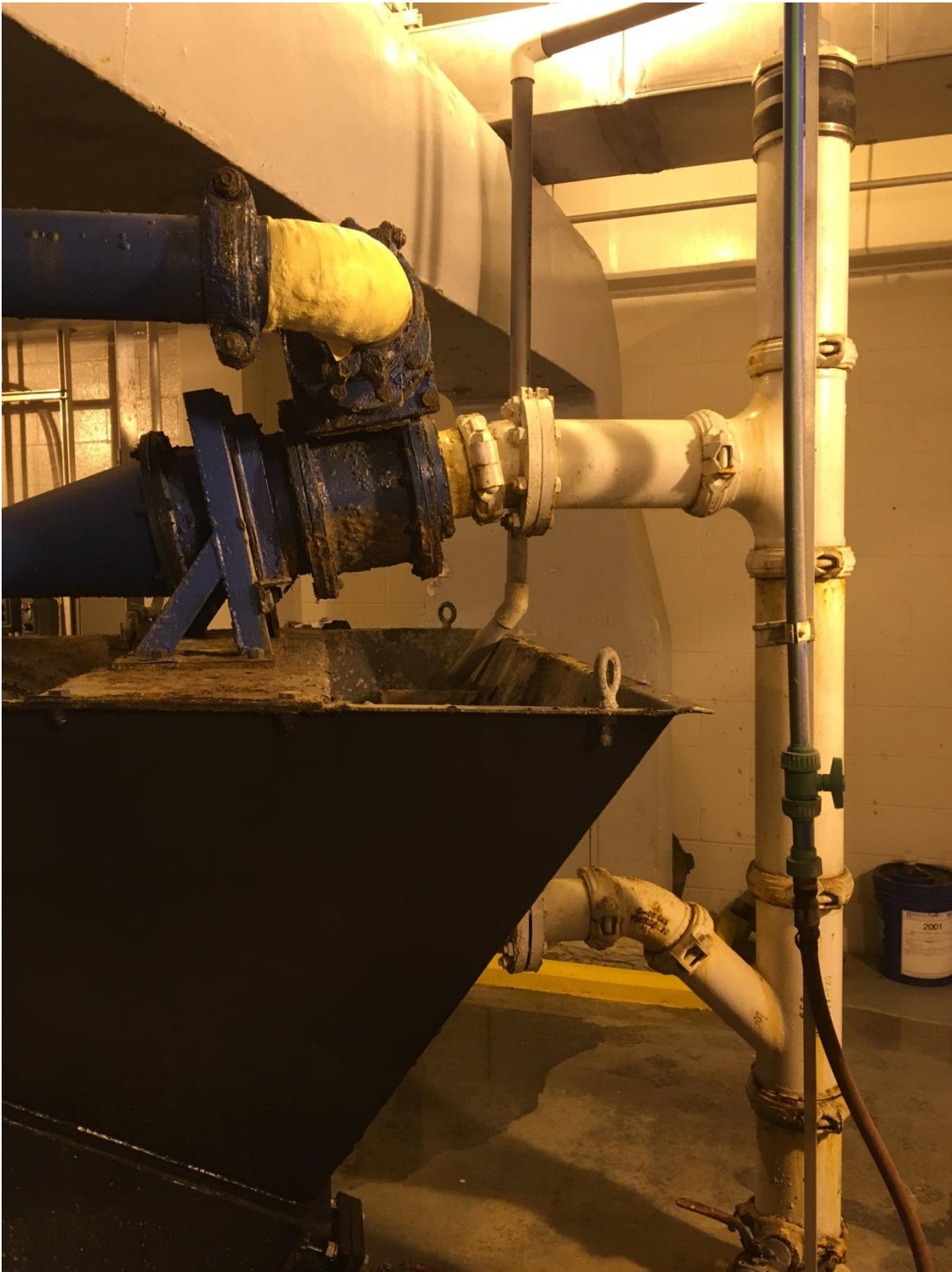
Figure 3: Grit Classifier H330 Discharge Piping & Vent
