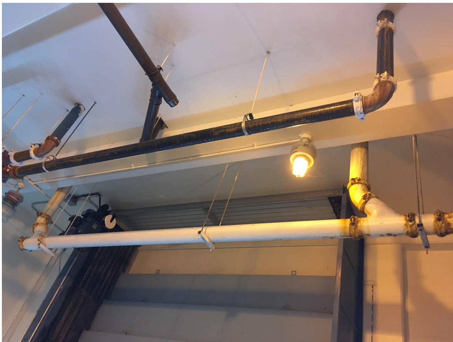
Figure 8: Intake (Black) & Discharge (White) piping
