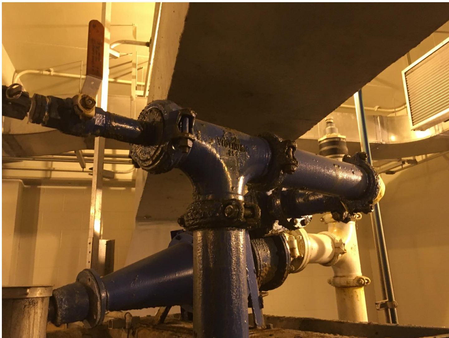
Figure 2: Grit Classifier H330 Intake Piping with Flushing Connection
