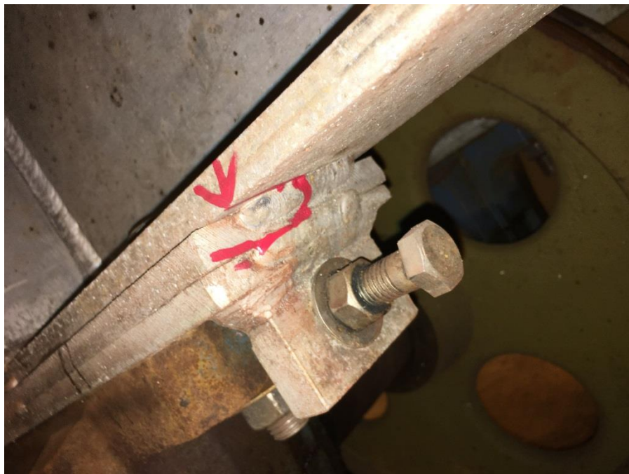
Cracked bearing mount plate weld at location 1B
