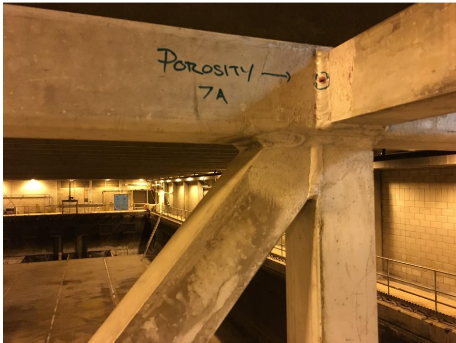
Porosity at location 7A
