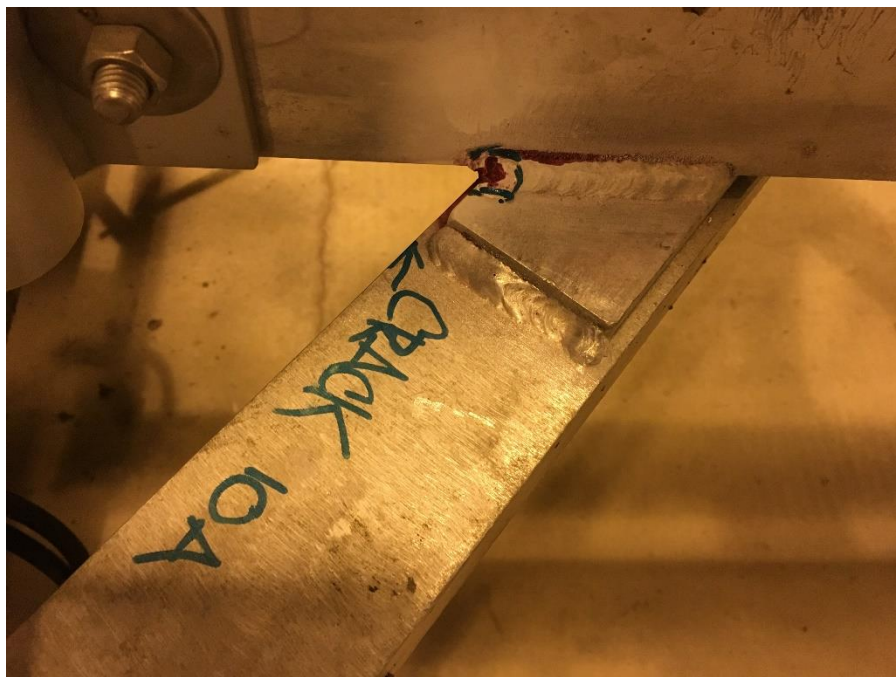
Crack at location 10A
