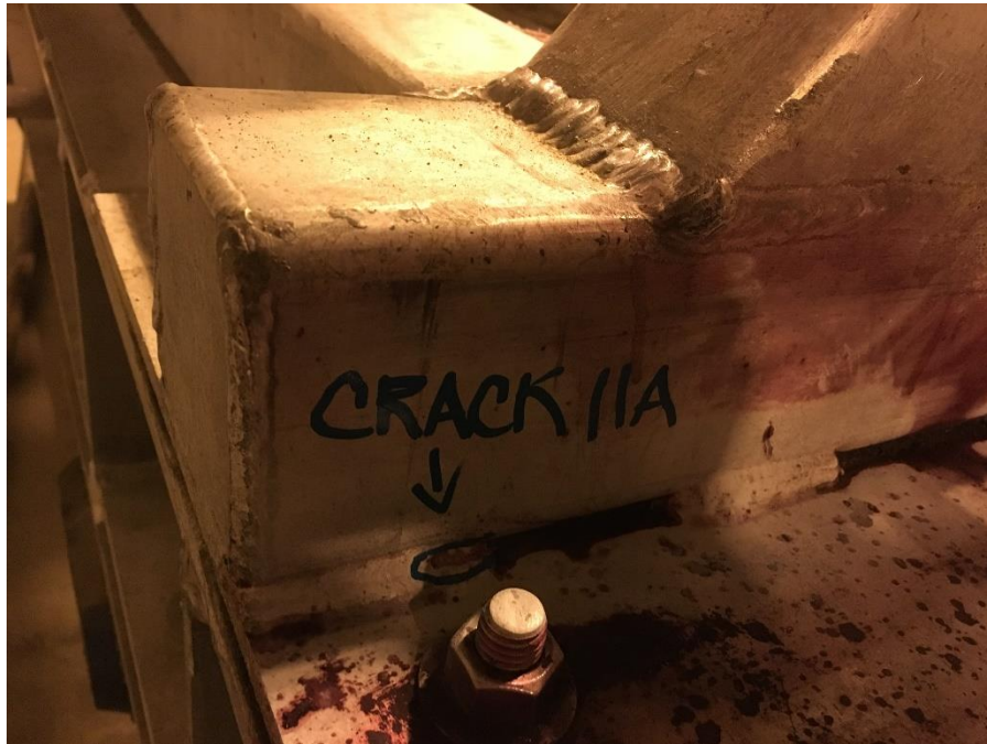
Crack at location 11A
