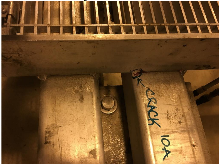
Crack at location 10A
