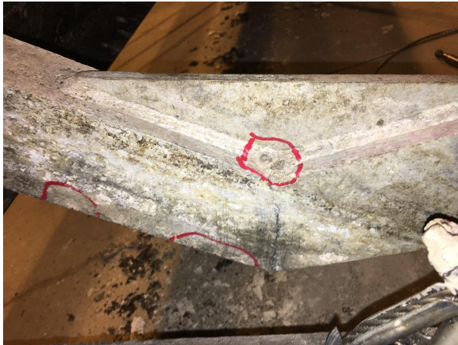
Photo showing pitted corrosion in scum paddle arm This is typical to all below water line aluminum members
