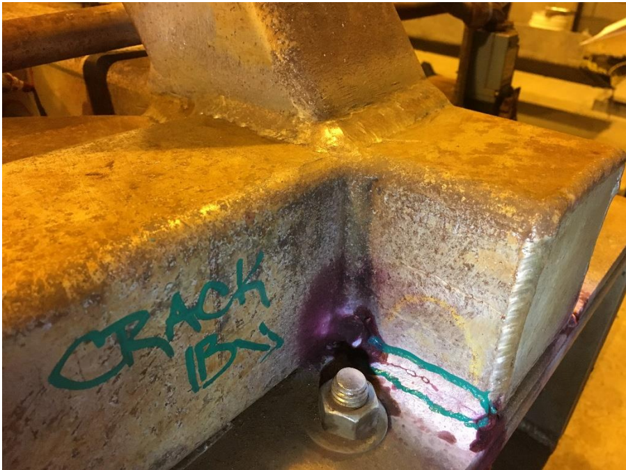
Crack at location 1B
