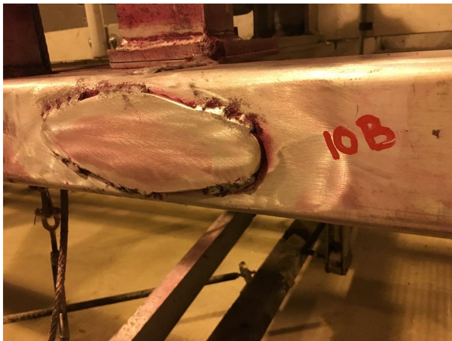
Photo of fish plate at location 10B. Poor weld quality
