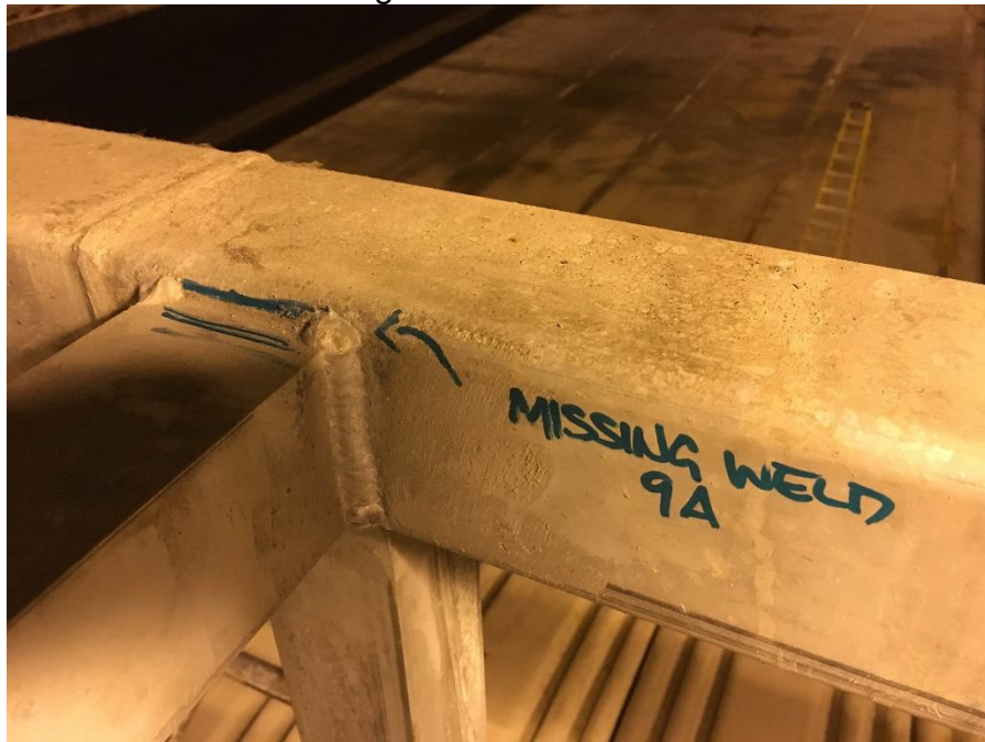
Missing Weld at location 9A
