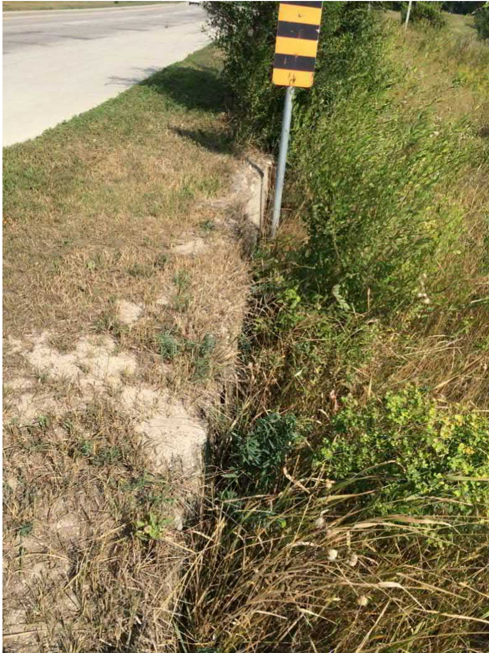
Subsidence of soil in front of retaining wall
