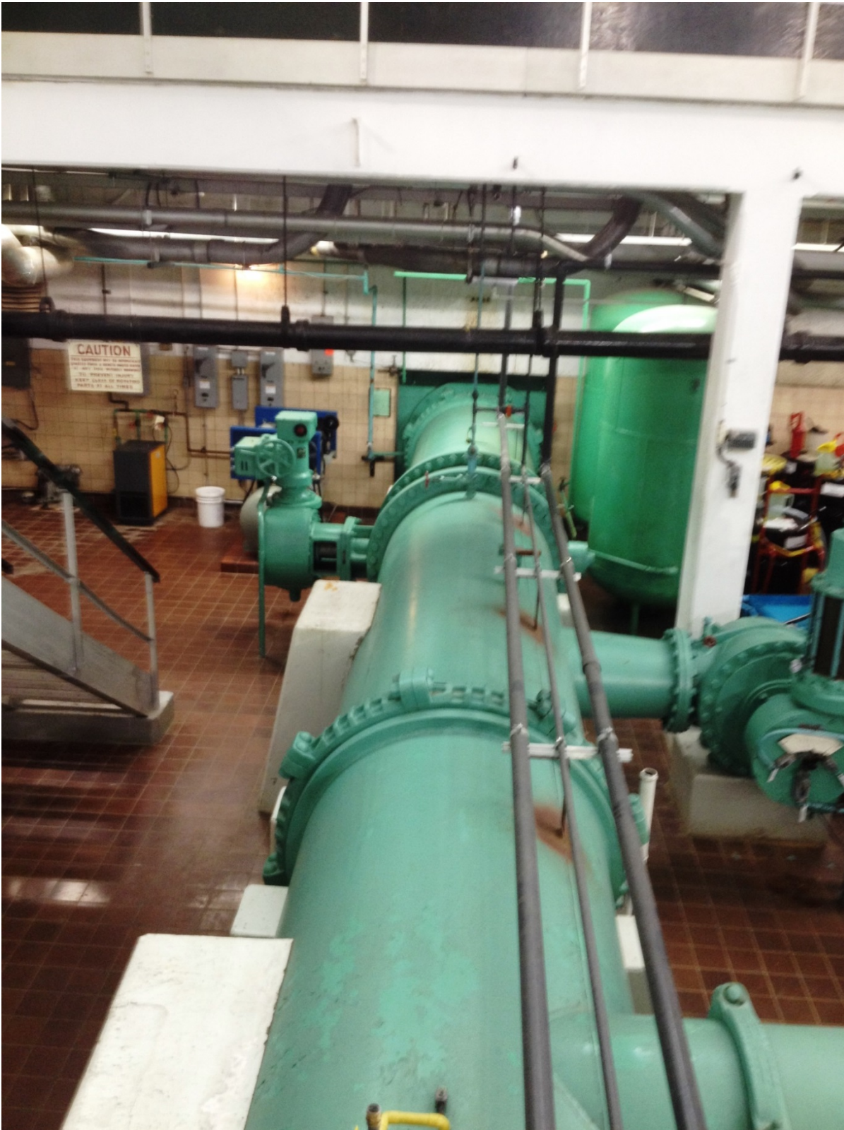
Photo 1: Hurst Discharge Header Looking East
