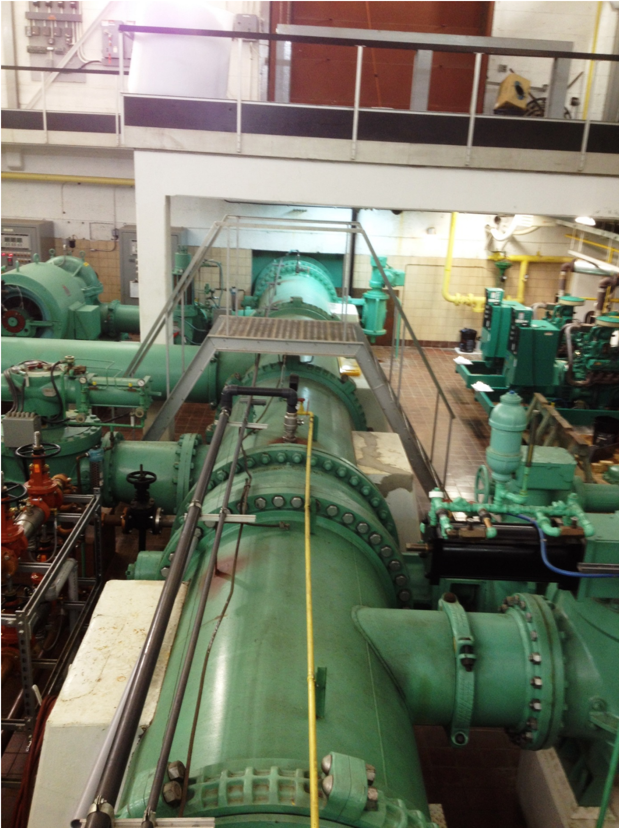
Photo 2: Hurst Discharge Header Looking West
