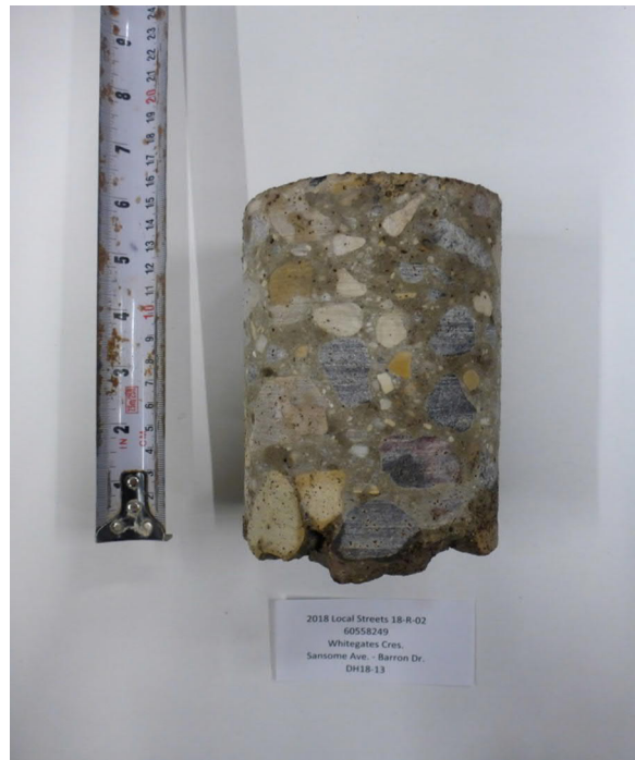
Photograph 22: Pavement Core PC18-23 – Whitegates Cresc
