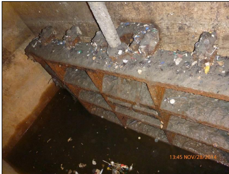
Photograph No. 9 Positive sluice gate
