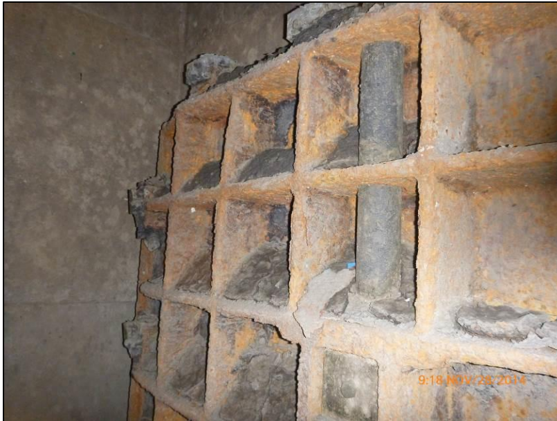
Photograph No. 9 Positive sluice gate
