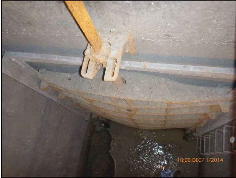
Photograph No. 9 Positive sluice gate
