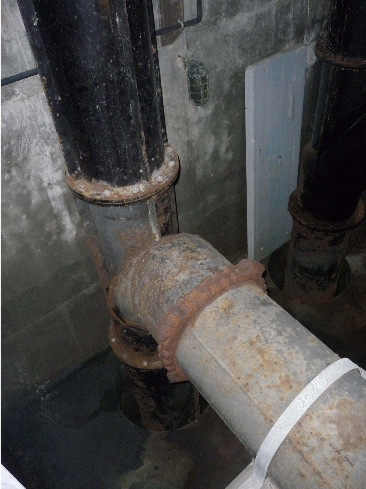
Figure 8: Metro Route 90 Underpass Pumping Station – Pump 1 Column Discharge
