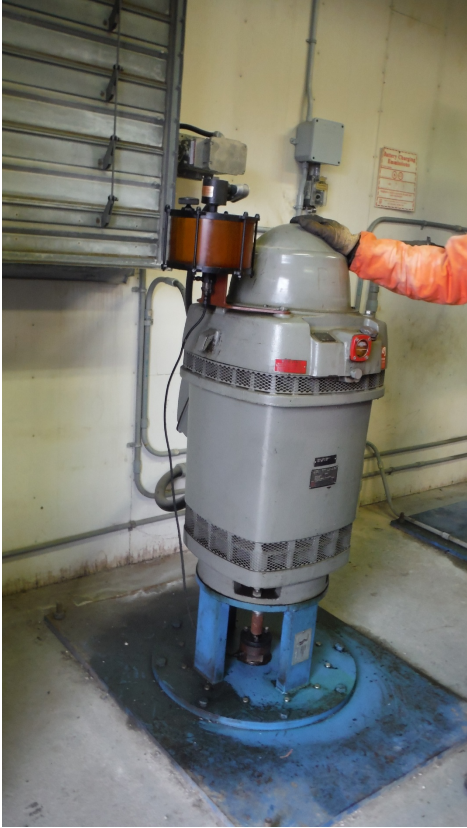
Figure 1: Metro Route 90 Underpass Pumping Station – Pump 1 Motor with Oil Lubricator (Top Left)
