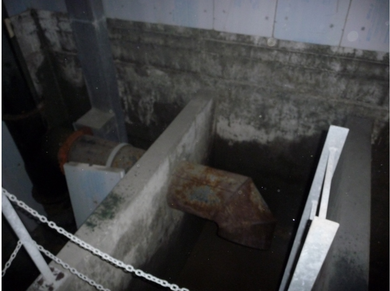
Figure 12: Metro Route 90 Underpass Pumping Station – Pump 2 Discharge Elbow
