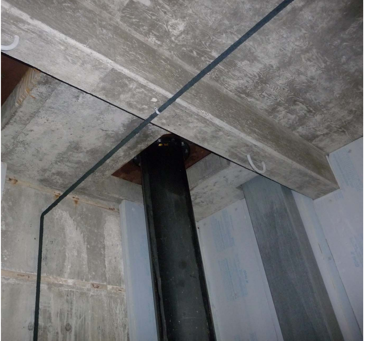
Figure 7: Metro Route 90 Underpass Pumping Station – Pump 2 Upper Column
