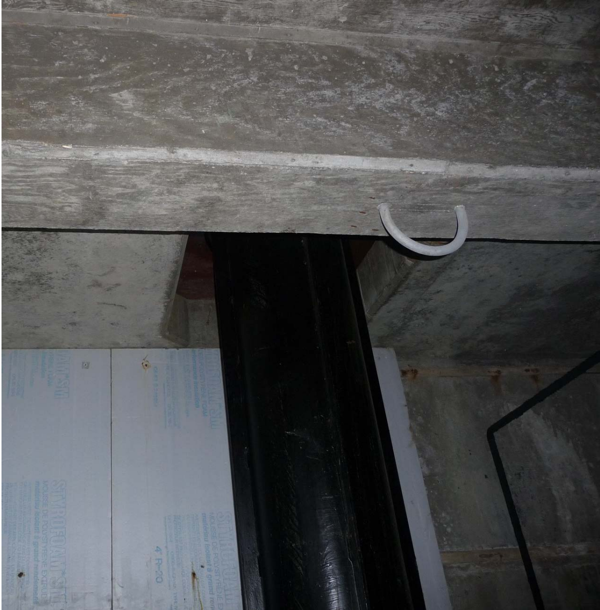
Figure 6: Metro Route 90 Underpass Pumping Station – Pump 1 Upper Column
