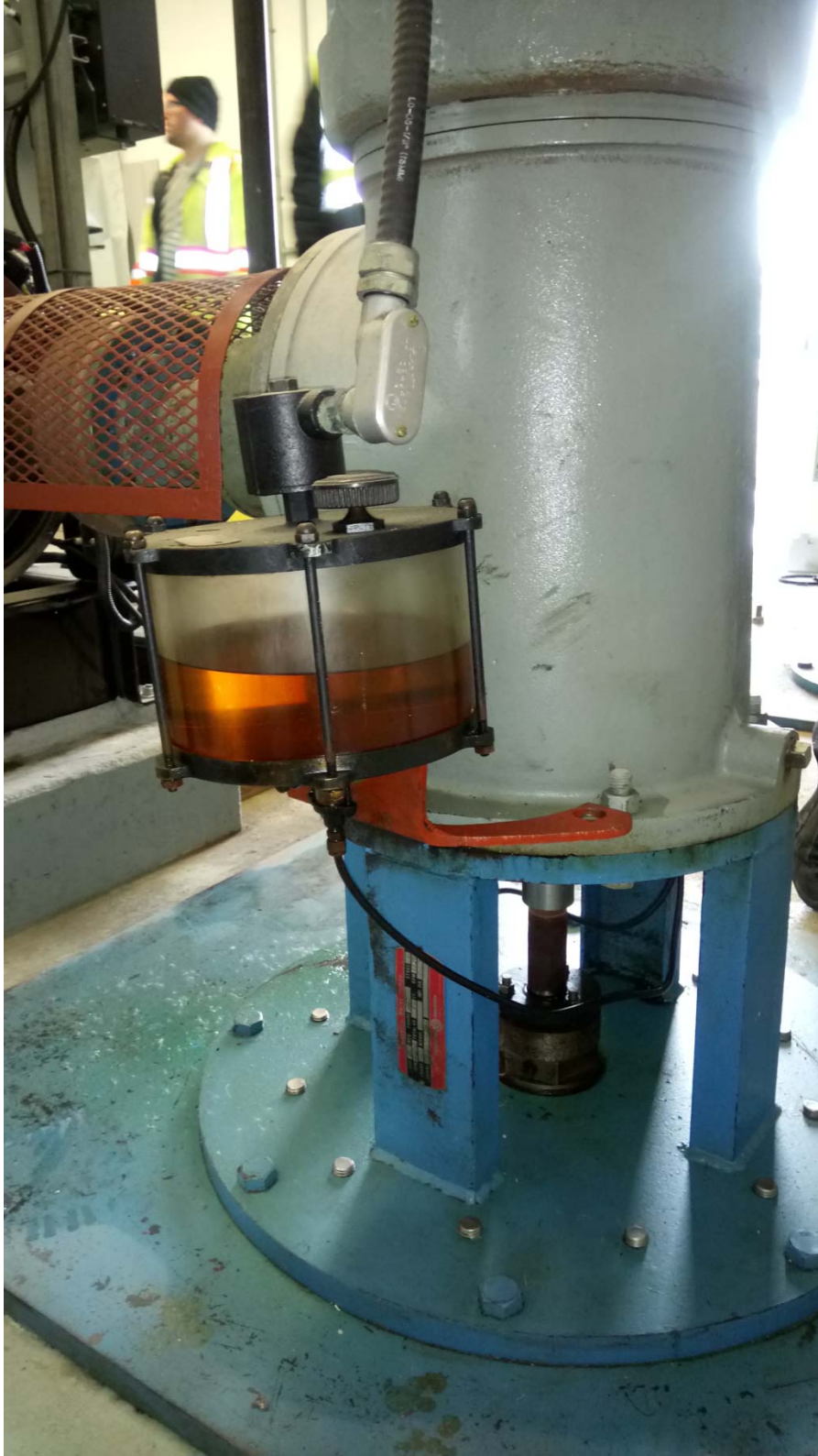
Figure 3: Metro Route 90 Underpass Pumping Station – Pump 2 Oil Lubricator
