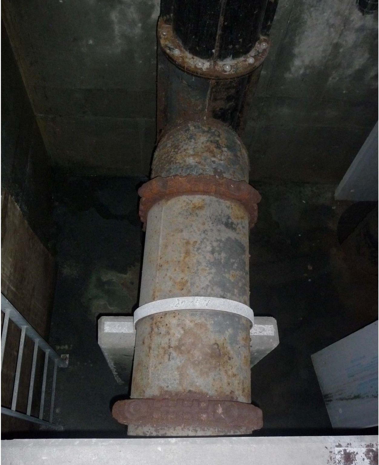
Figure 9: Metro Route 90 Underpass Pumping Station – Pump 1 Horizontal Discharge Piping
