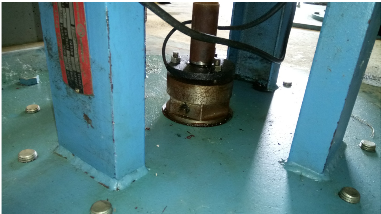
Figure 5: Metro Route 90 Underpass Pumping Station – Bearing / Packing
