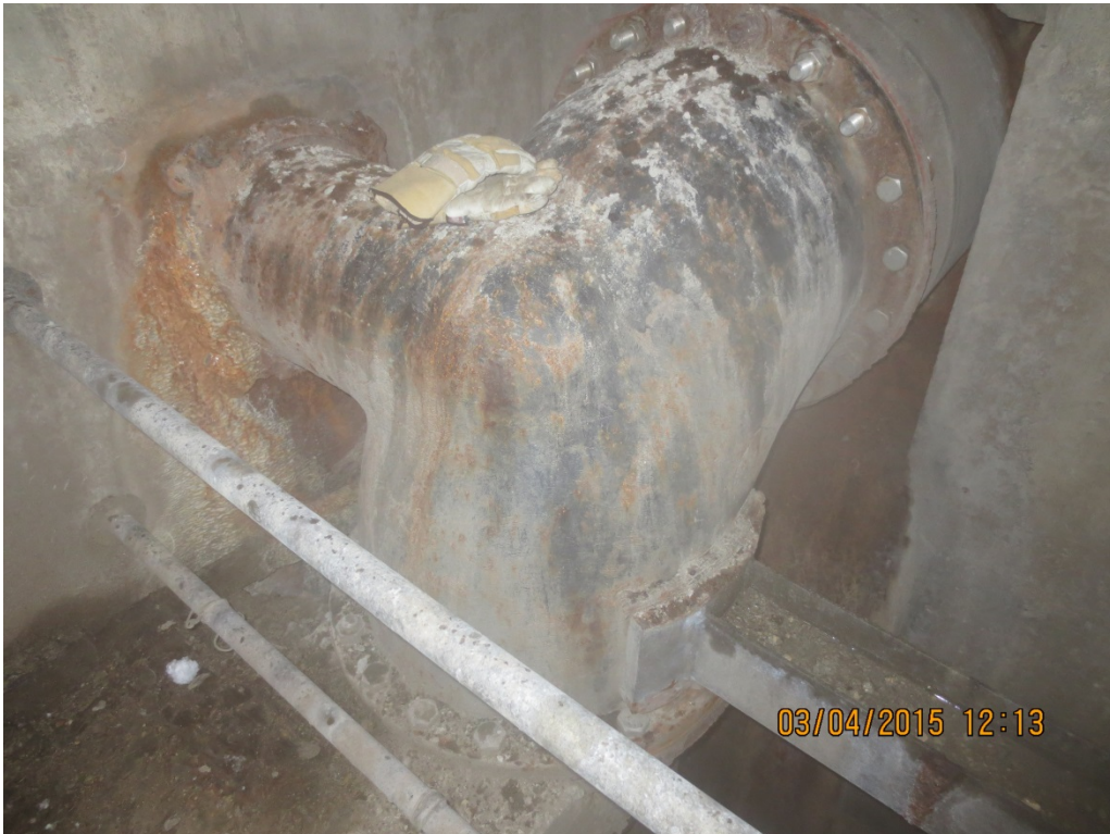
Site 1 – West chamber interior - existing side-outlet elbow with welded brace
