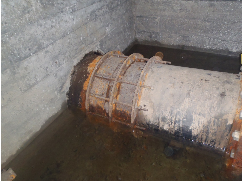
Site 1 – East chamber interior - 600 feeder main
