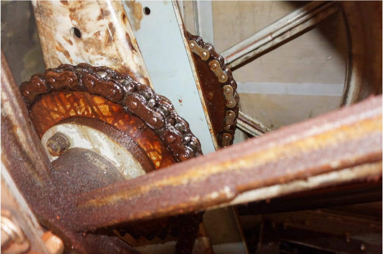
The handrail drive chain in the foreground is worn out (down escalator). Chain in background is up escalator handrail drive chain (newer).
