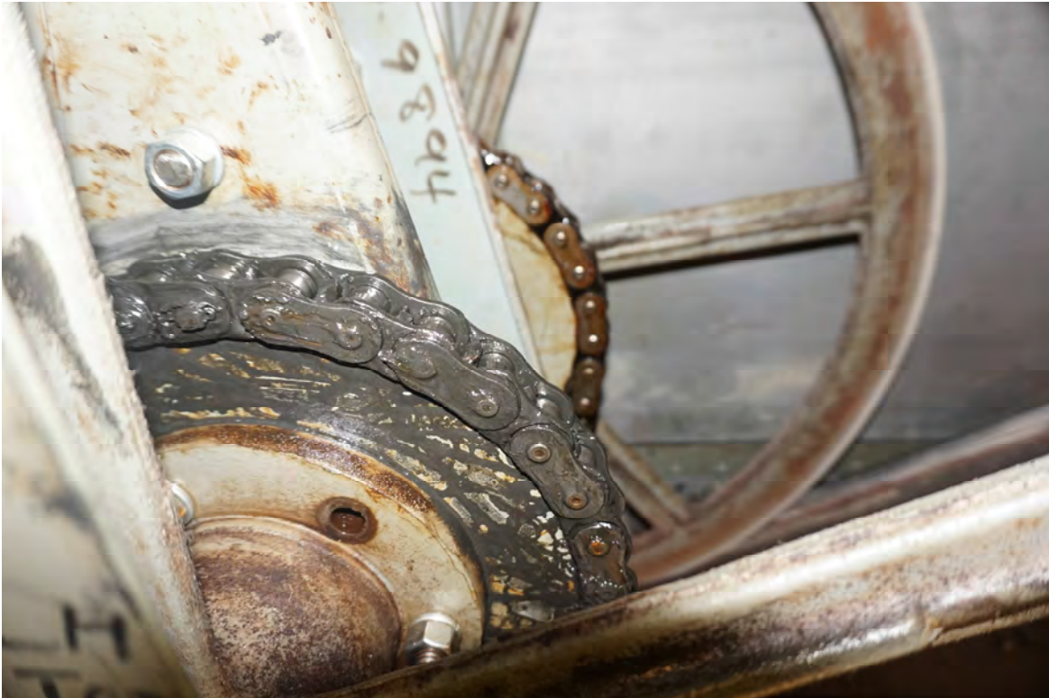
Down escalator handrail drive chain
