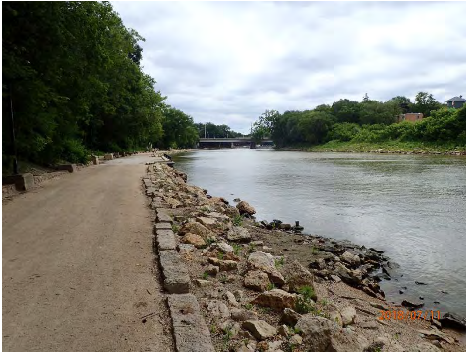
Photo 7 – Looking downstream (NE) at exposed riprap protection along the River Walk lower berm shoulder at the approximate alignment of the Donald Outfall.
