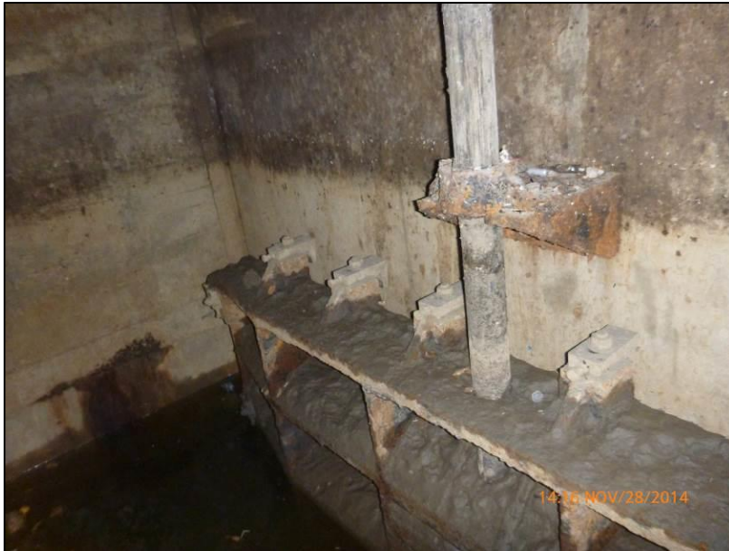
Photograph No. 9 Positive sluice gate
