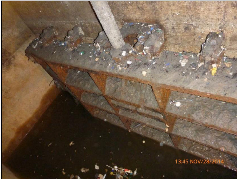
Photograph No. 9 Positive sluice gate
