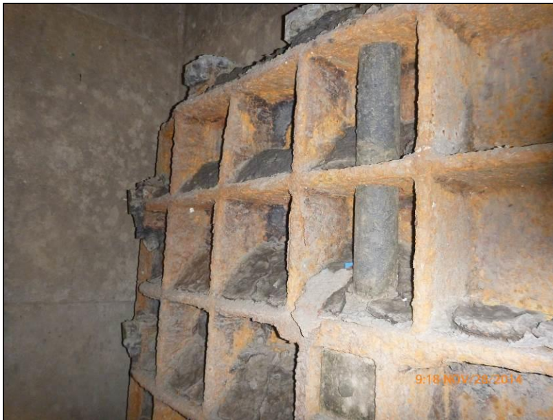
Photograph No. 9 Positive sluice gate
