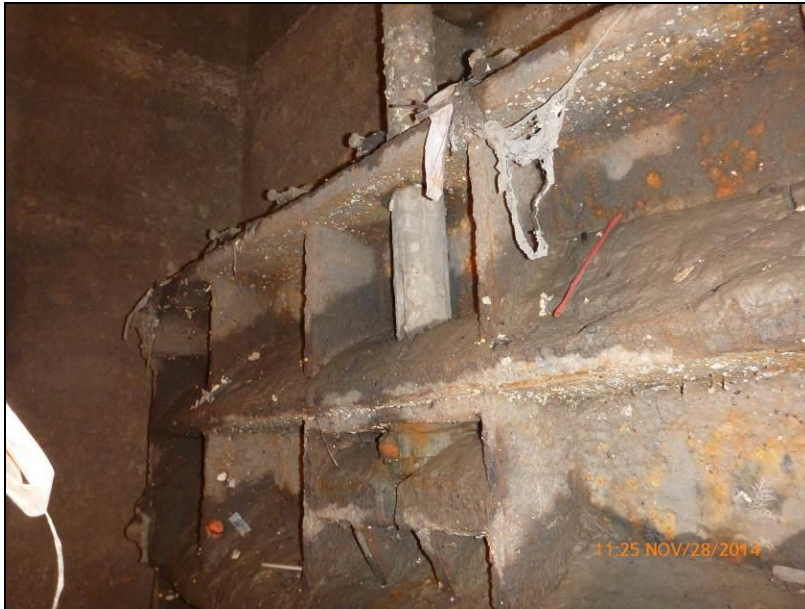
Photograph No. 9 Positive sluice gate
