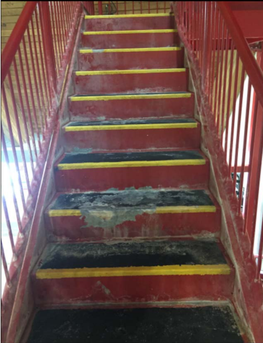
Image 5: Front Top View of Deteriorated Stair Treads/Risers
