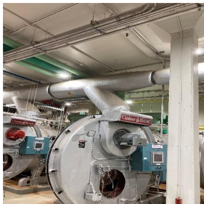
Asbestos-containing parging cement present on mechanical equipment in various locations in GOOD condition.
