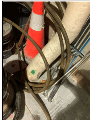
Damaged/exposed parping cement on 3 rainwater leader fittings within Location No.12.
