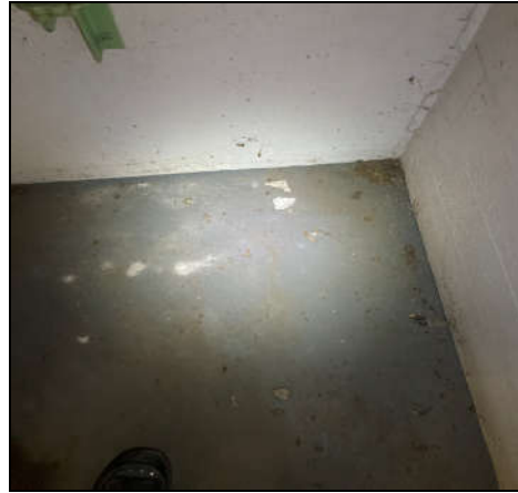
Parging cement debris Location No.33
