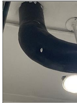
Damaged/exposed parging cement within the Chlorine Building, Chlorinator Room, Location No.9
