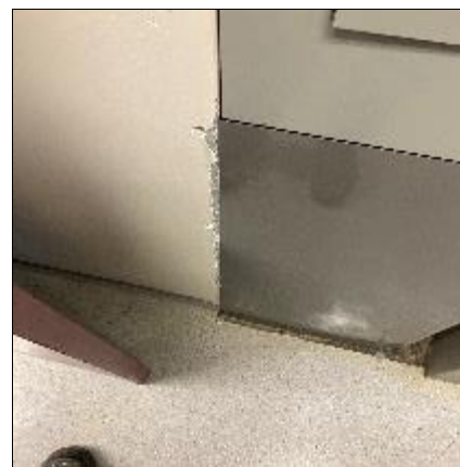
Damaged drywall joint compound, Location No.26
