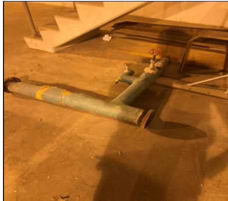
Parging cement debris present on cut section of pipe within Location No.30
