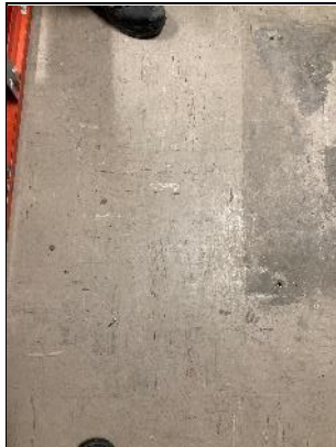
Asbestos-containing vinyl floor tiles within Electrical Room Location No.6.
