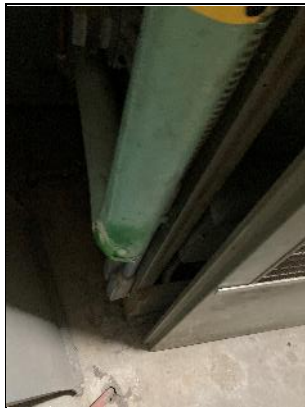
Damaged/exposed parging cement within the Old Pump Building Furnace Room Location No.21
