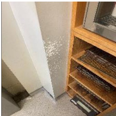
Damaged drywall joint compound, Location No.26
