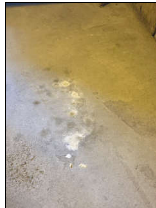
Parging cement debris present under the damaged ducting within Location No.'s 6 and 7.
