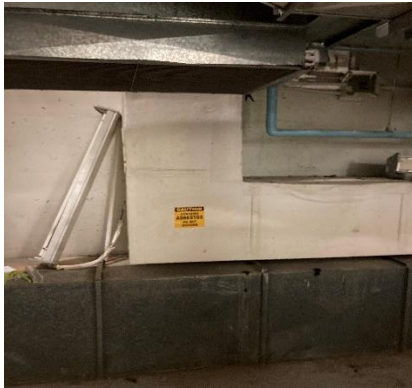
Asbestos containing parging cement insulating ducting in various location observed in good condition.
