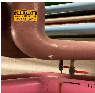
Damaged/exposed parging cement on 3 fittings within the Grit Building Location No. 59.
