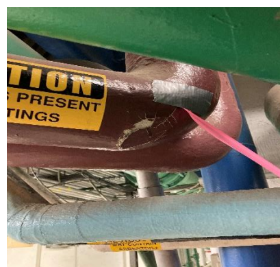
Damaged/exposed parging cement on 3 fittings within the Grit Building Location No. 59.
