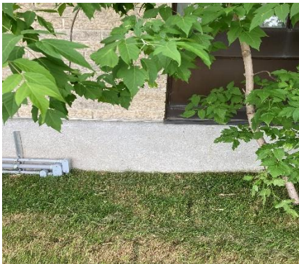
Presumed and confirmed asbestos-containing plaster in various locations observed in GOOD condition.
