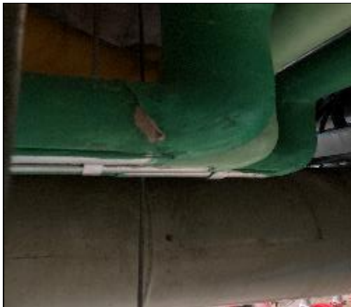
Damaged/exposed parging cement in FAIR Condition, Location No,34.
