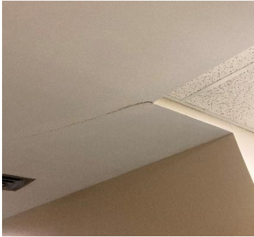
Damaged asbestos-containing drywall joint compound in FAIR condition within the Admin Building Location No.11.
