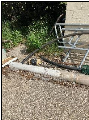
Asbestos-containing transite cement pipe debris exterior of Garage Building F..
