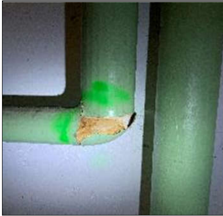
Damaged/exposed parging cement Location No.33
