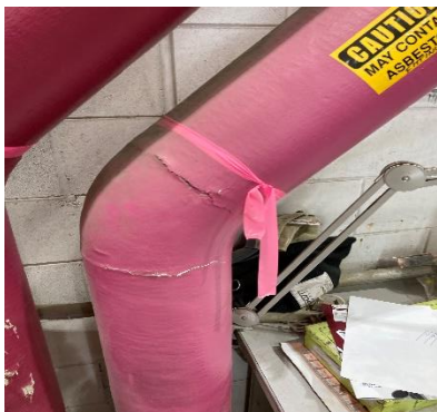
Damaged/exposed parging cement on 1 fitting within the Service Building Location No. 68.
