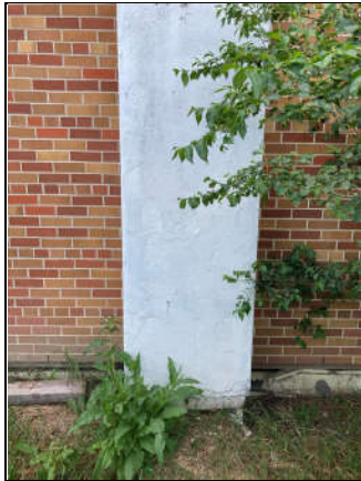
Asbestos-containing plaster present on exterior wall.
