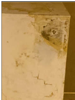
Damaged/exposed parging cement on intake ducting within Location No.'s 6 and 7
