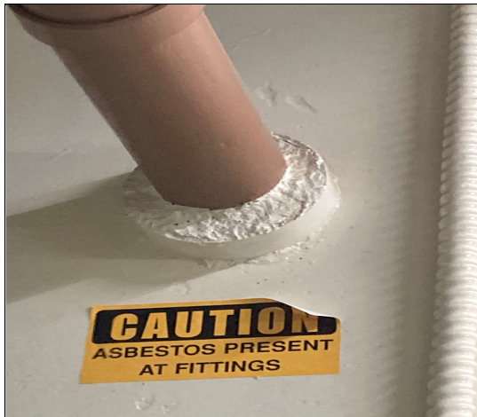
Asbestos-containing parging cement present as firestop.
