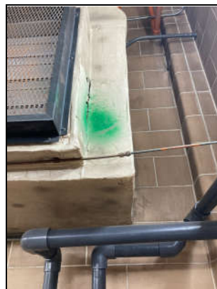
Damaged/exposed parping cement on 1 SF of ducting within Location No.6.
