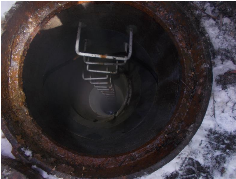
Conway Wet Well
