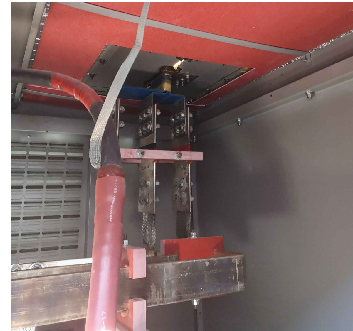
LST-4 SECONDARY BUSDUCT CONNECTION
